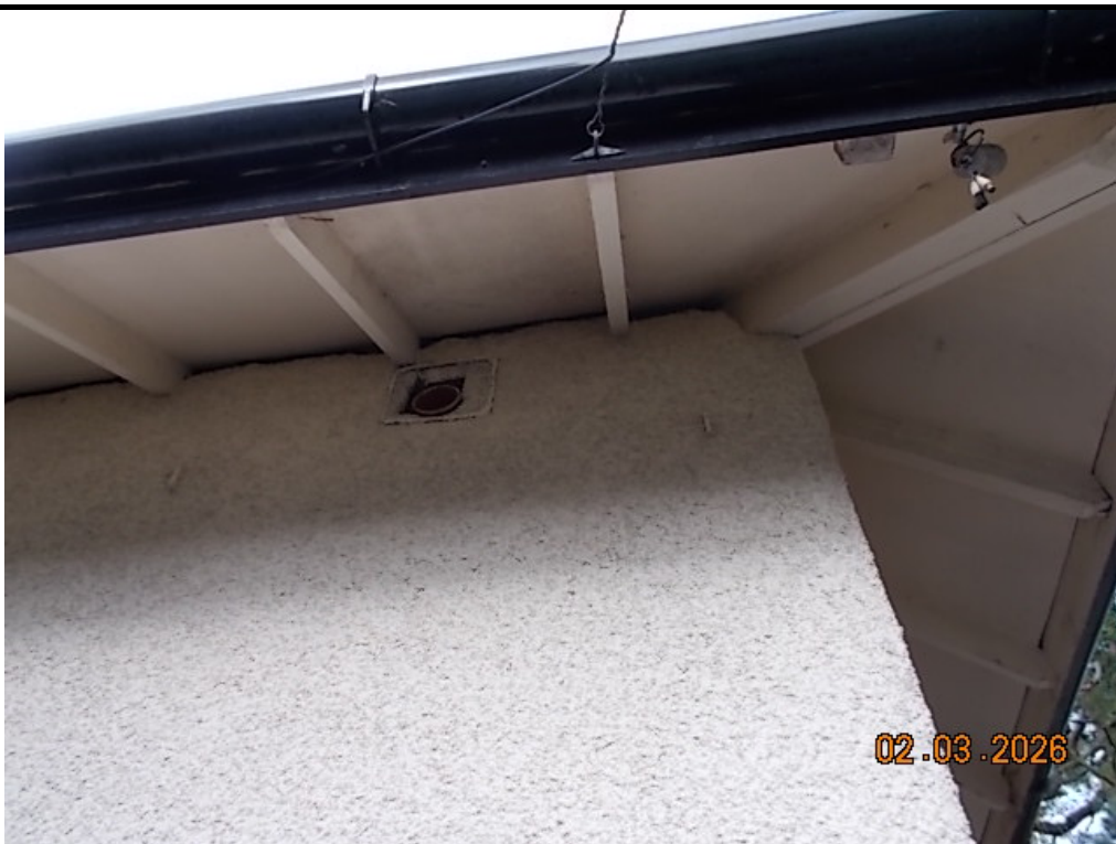
32. Kitchen extract fan external
