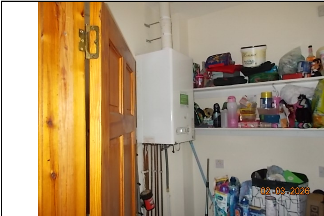
7. Utility Room with boiler
