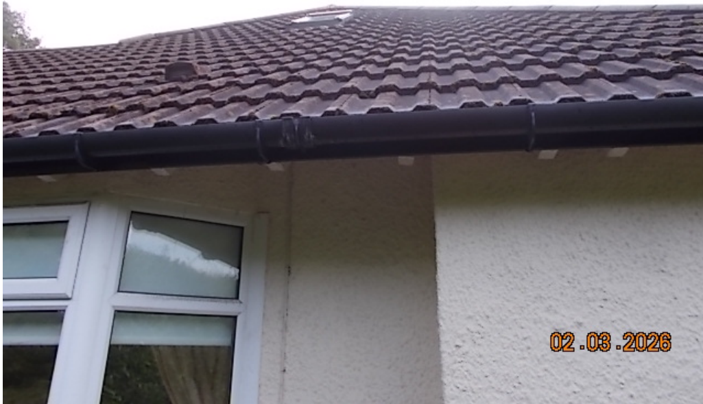
29. Side gutter with leaking joint
