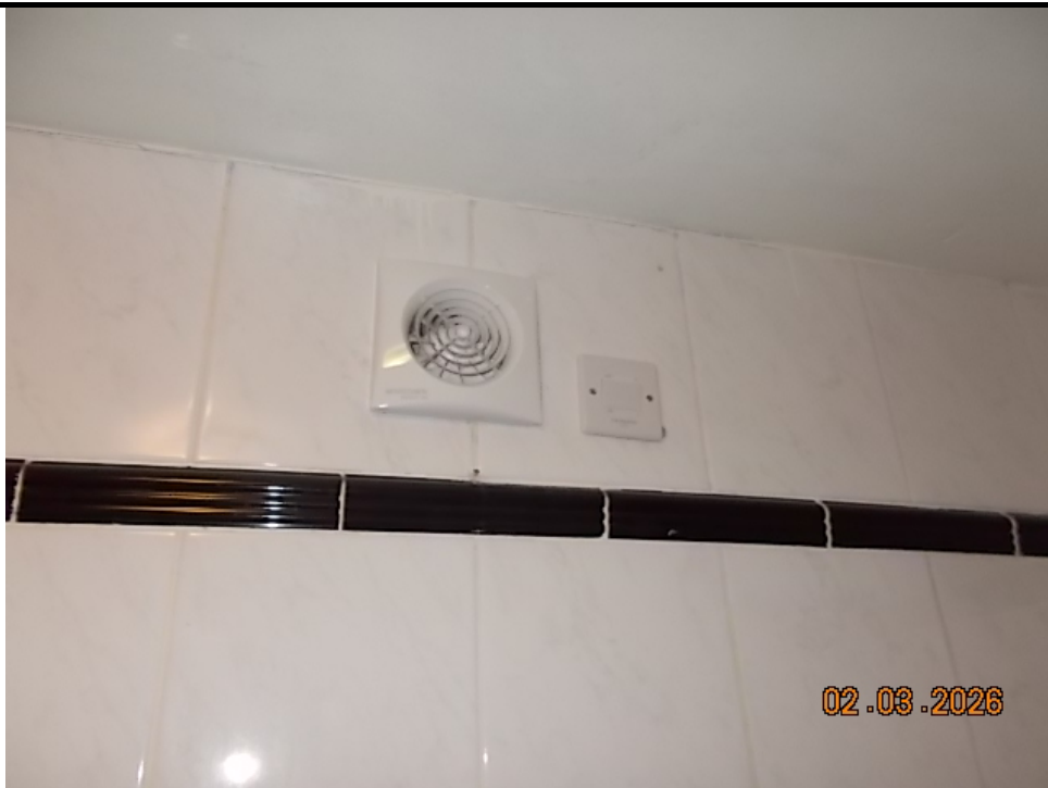
8. Extract fan in family bathroom
