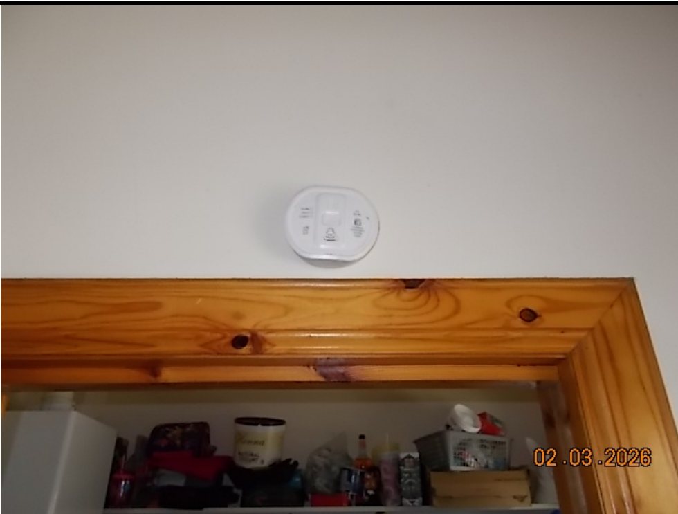
6. Carbon Monoxide Alarm above door from Kitchen to Utility Room
