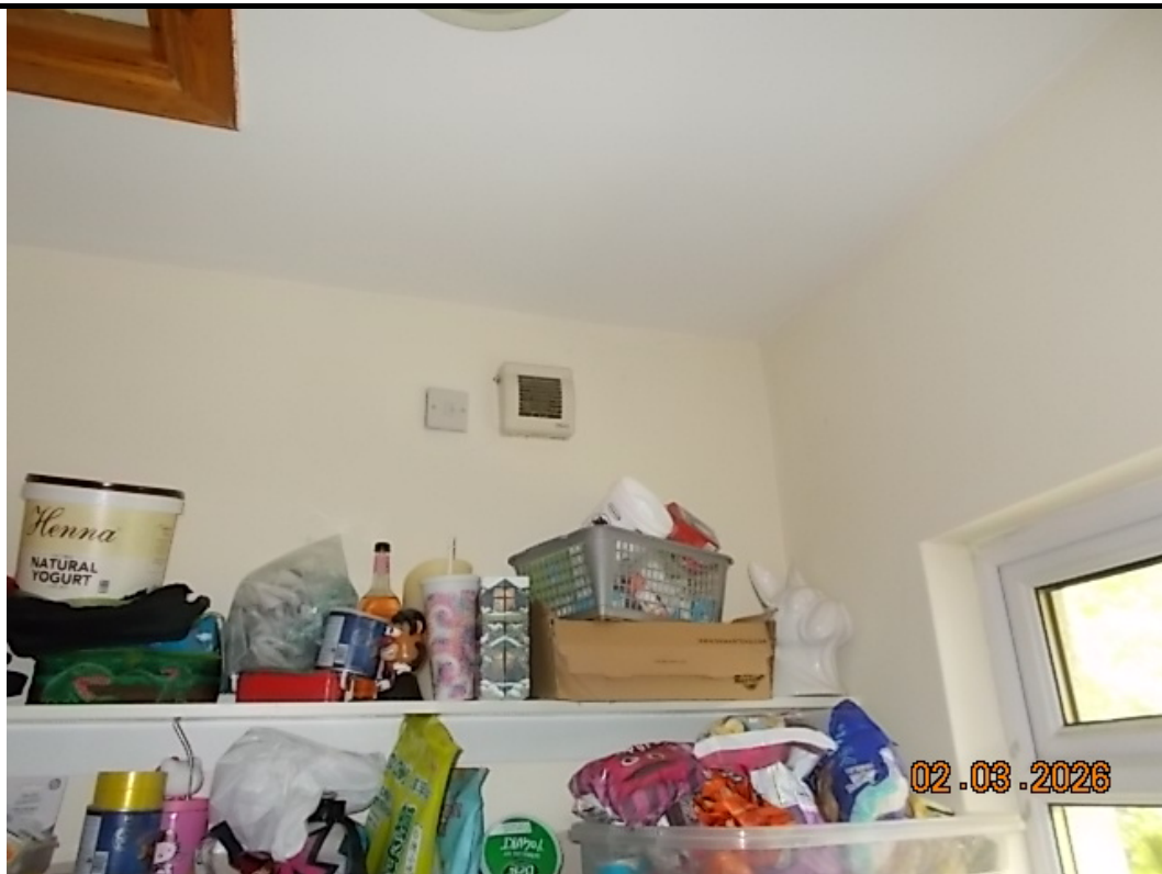
16. Extract Fan in Utility Room
