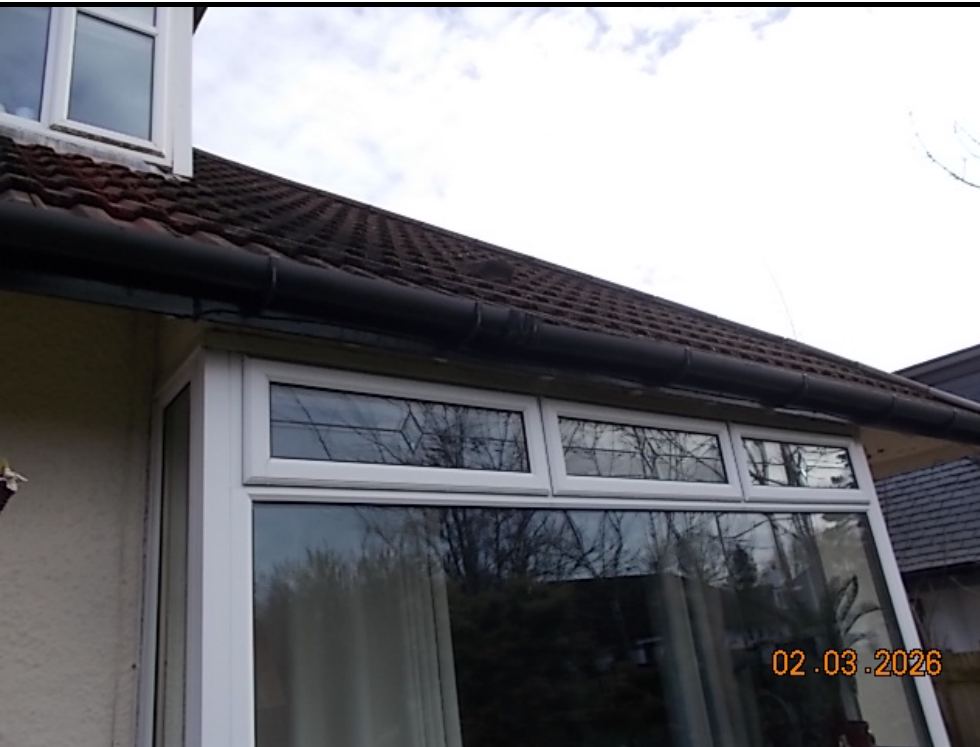
26. Front Gutter with leaking joint
