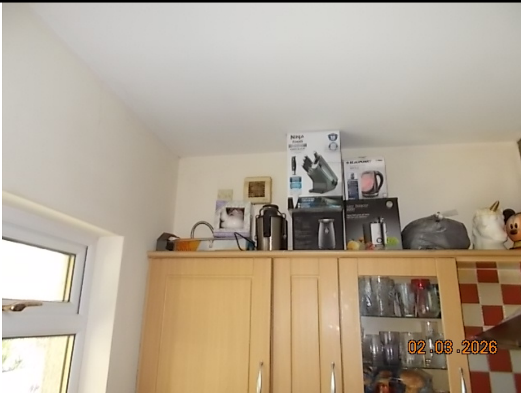
17. Extract Fan in Kitchen
