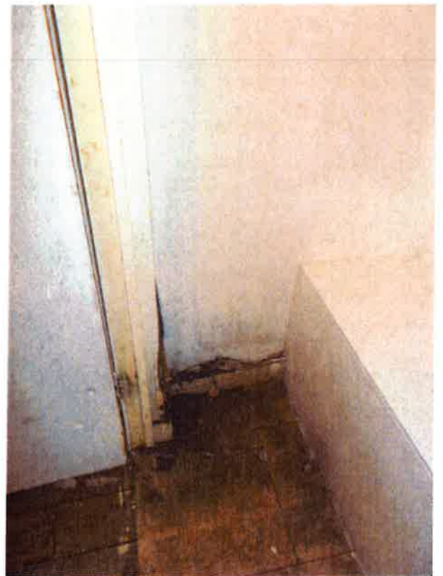
1. (e) Cupboard 1st floor off landing adjacent to room with boiler
