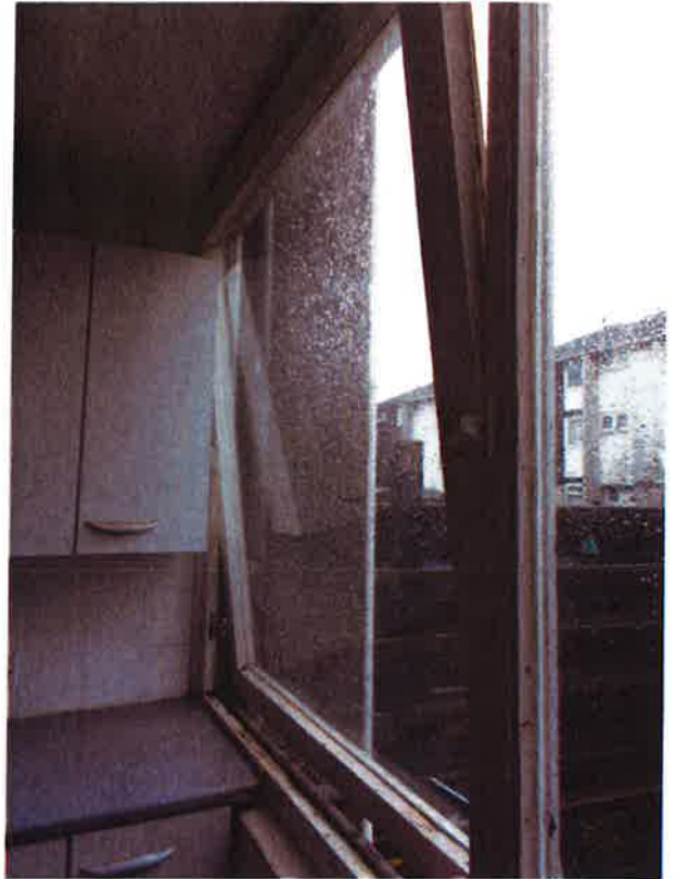
1. (f) Kitchen window on left opens but restricted by kitchen cupboards
