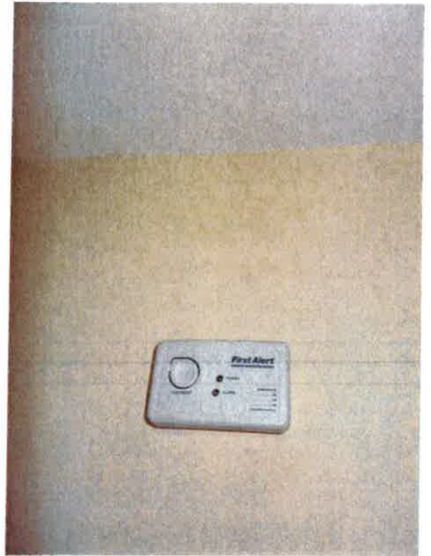
3. Carbon monoxide alarm - 1st floor left room
