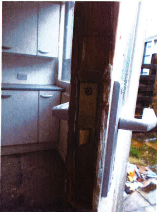
1. (j) Wood split to back door at new mortice lock
