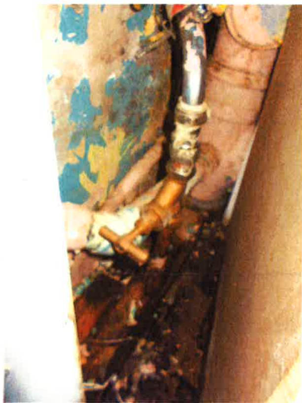
2. GF cloaks - pipe leaking behind boxing
