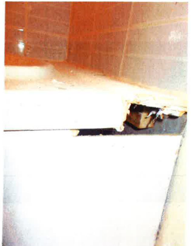
16. Bath - gap at panel/sealant/wall
