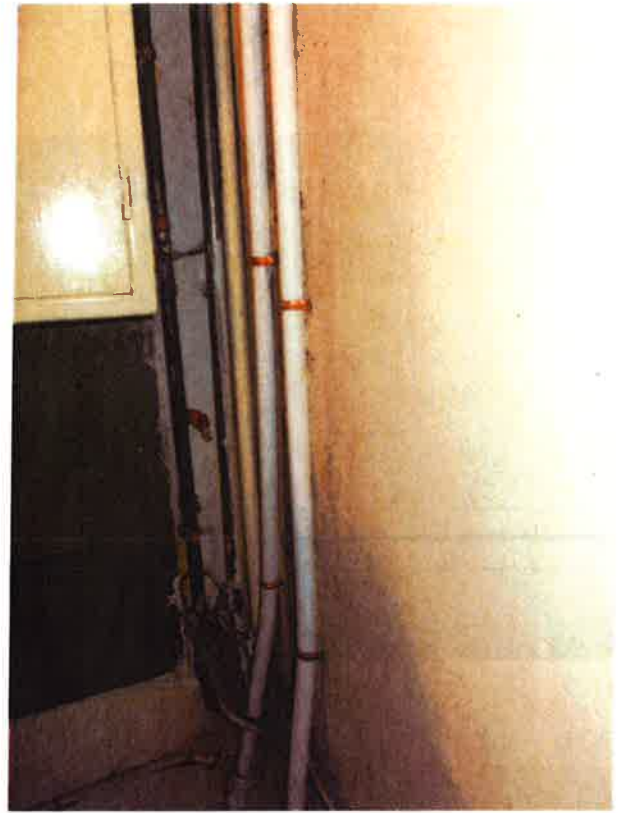
2. Ground floor meter cupboard
