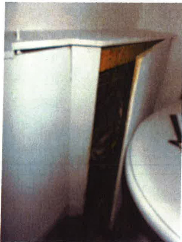
1. GF Cloaks - boxed pipes/exposed screws
