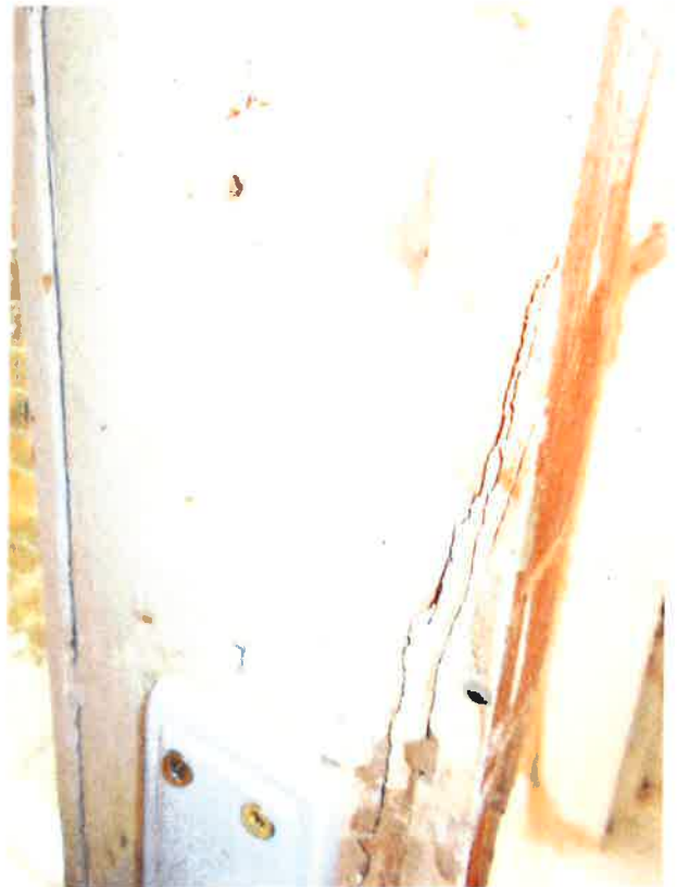
1. (j) Wood split to back door at new mortice lock
