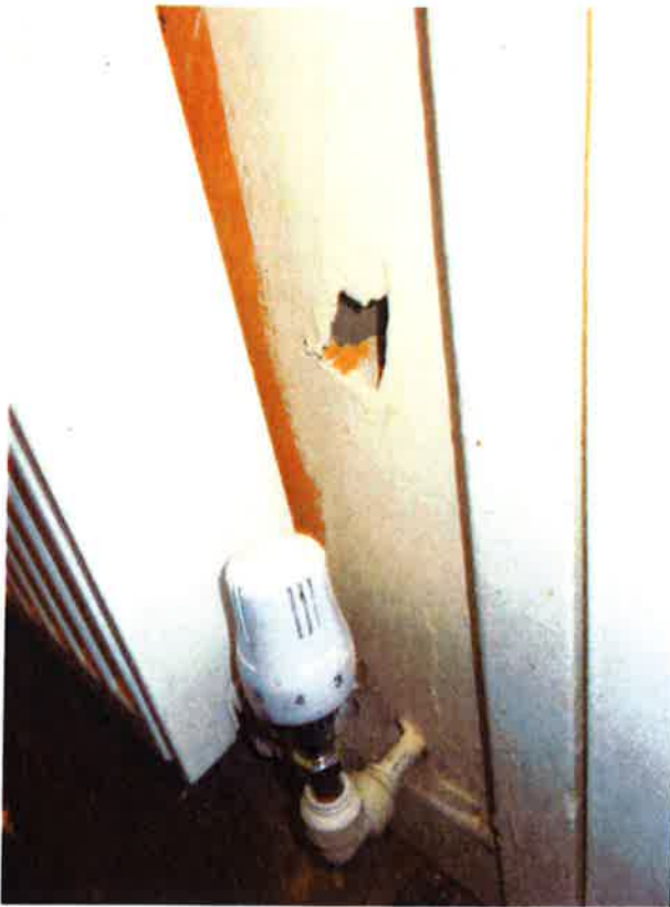
33. GF Hall - Pipe secure but hole in plasterboard wall
