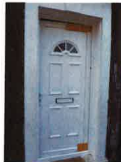
9. Damaged replacement front door
