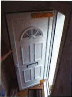
8. Damaged replacement front door
