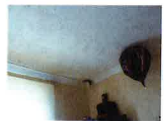
13. Plaster/decoration at water damaged bedroom
