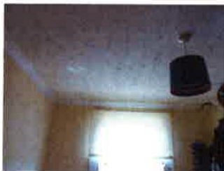
11. Plaster/decoration at water damaged bedroom
