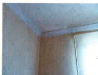
12. Plaster/decoration at water damaged bedroom
