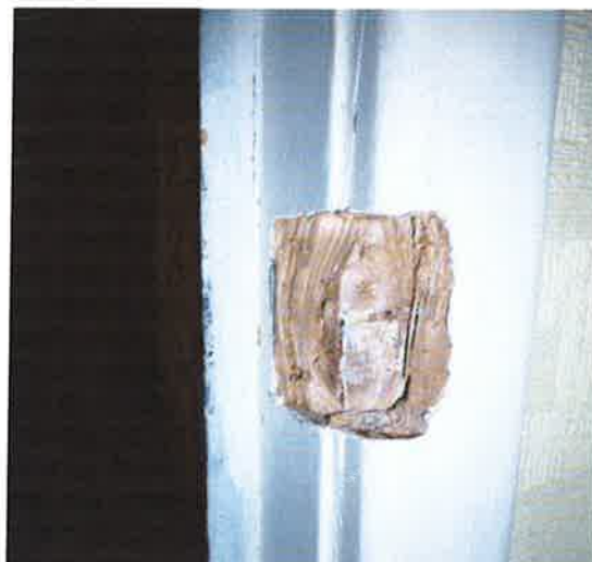
Missing keep – door insecure
