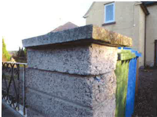
Loose concrete coping stones to front gates
