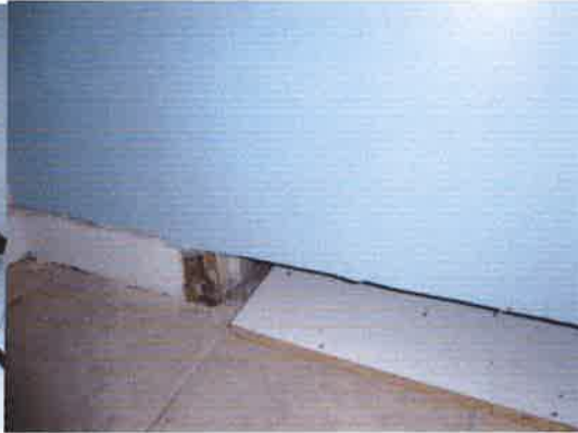
Kitchen – no skirtings in room
