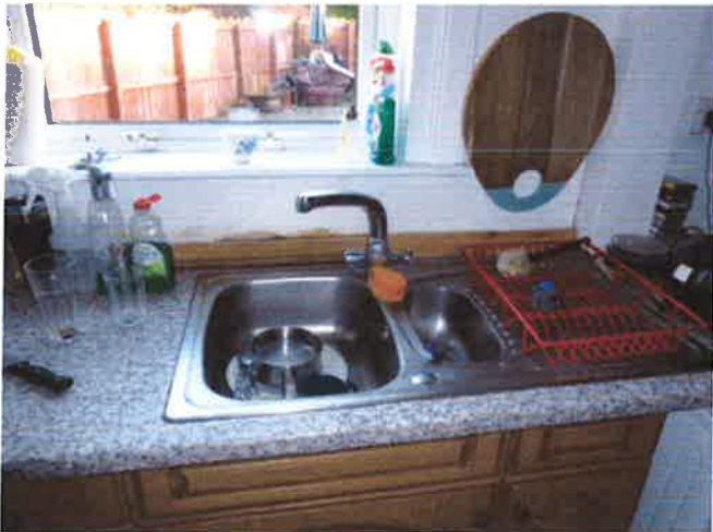
Kitchen sink – no plug and chain
