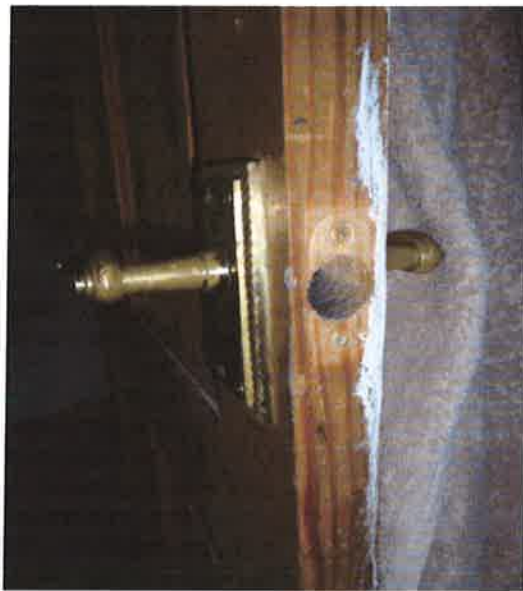
Holes where door latch should be
