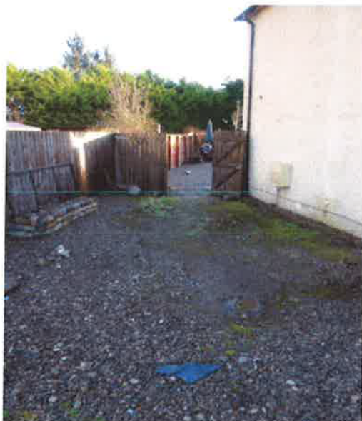
Flooding area around gas meter
