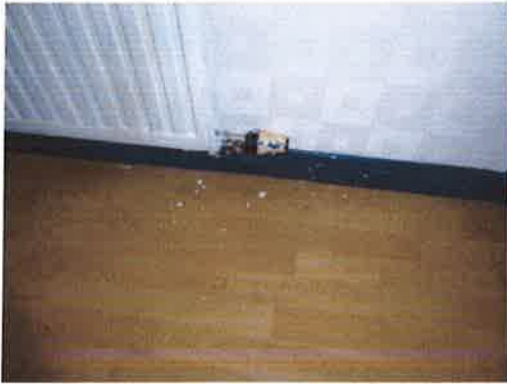
Central heating radiator
