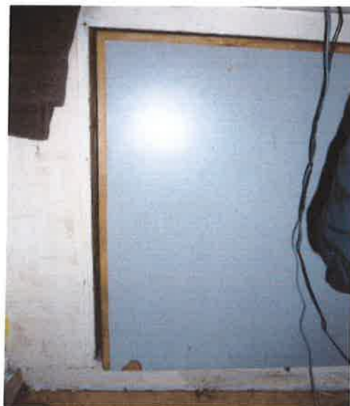
Electric meter cupboard – ill-fitting door
