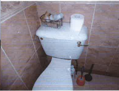
First floor WC and Cistern
