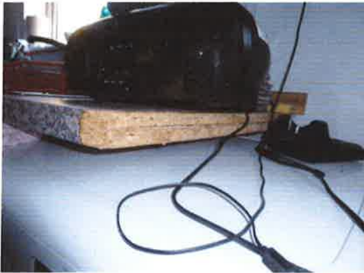
Kitchen worktops – exposed bare timber – missing iron-on edging strips
