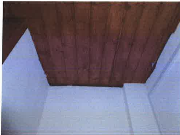
Ceiling – missing quadrant beading around perimeter
