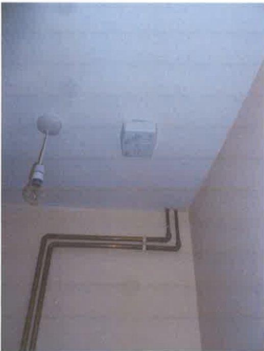
CO Detector Boiler Cupboard- April 2018
