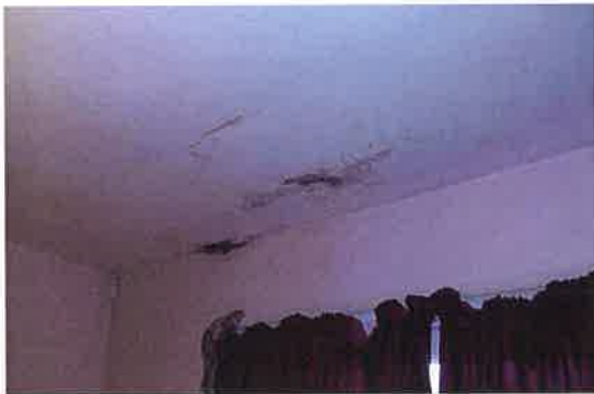
Photo 6 – Main bedroom ceiling
