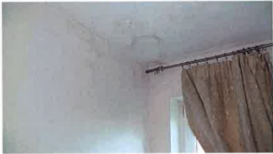
Photo 2 – Water damage in living room (L/H)
