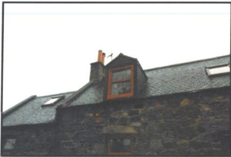
Figure 5 Front elevation left hand side - all guttering replaced, replacement windows, replacement chimney cans.
