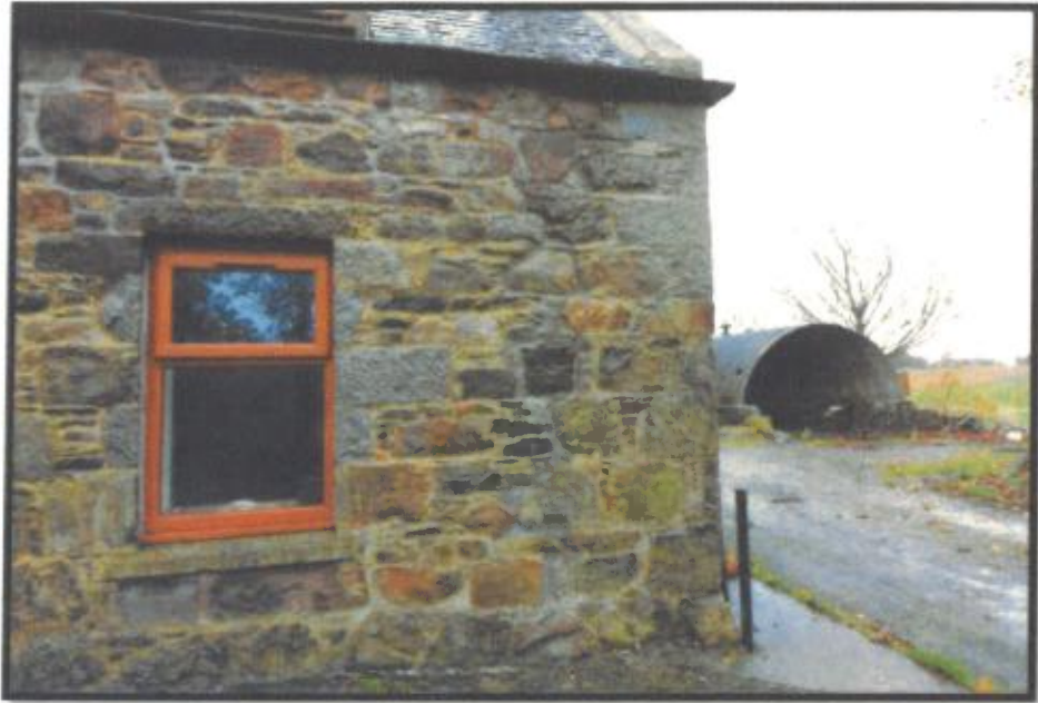
Figure 4 Front elevation right hand side vertical crack re-pointed, window replaced.
