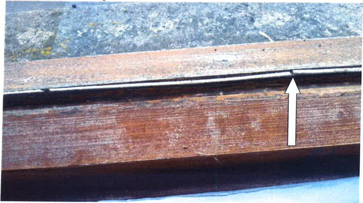
8. Close view of glazing putties which are cracked and generally detached from timber beads..
