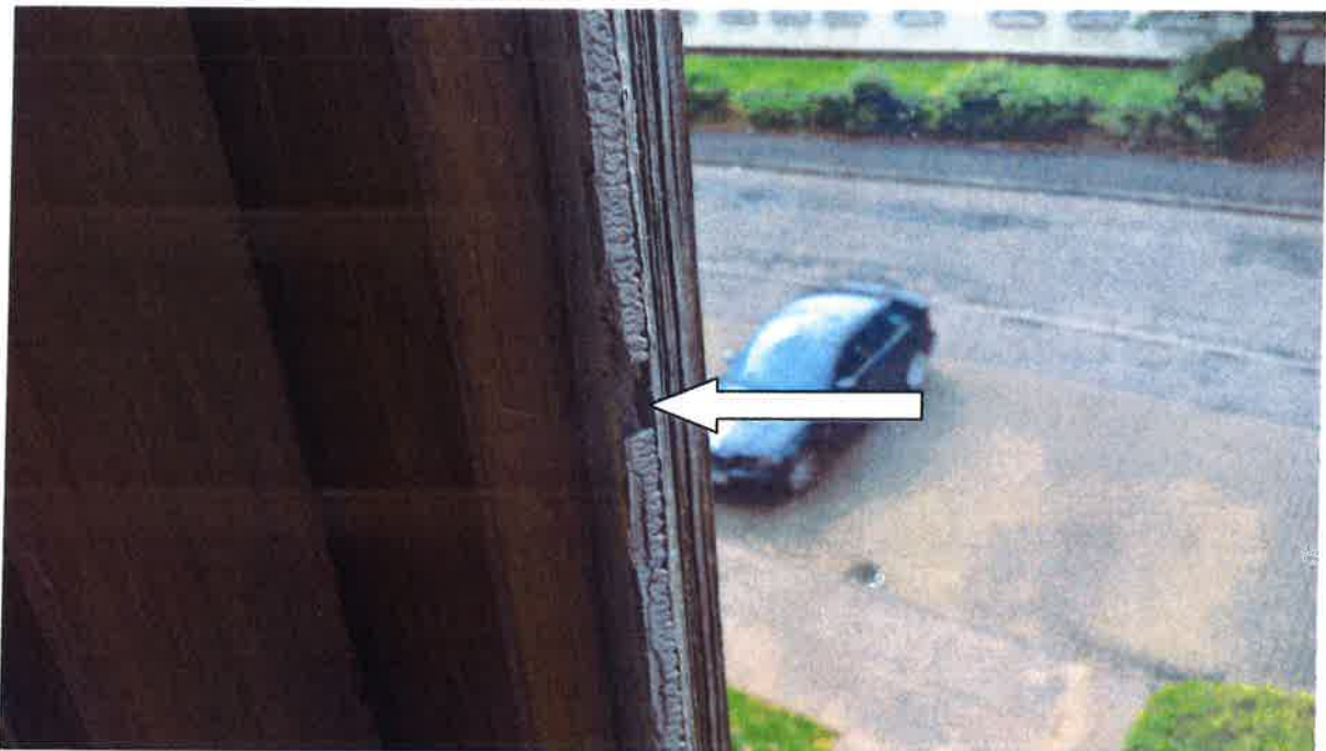
1. Close view of defective glazing putty providing weatherseal.
