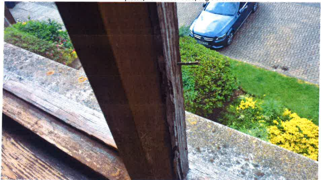
6. Further view of loose timber trim to external glazing seal.
