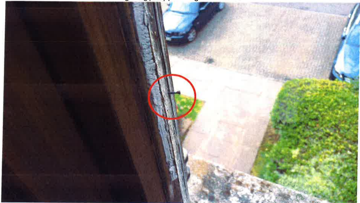
2. View of cracked and perished glazing putty and loose timber trim with pins projecting.
