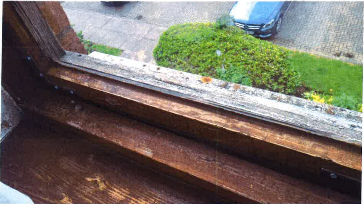
3. View of remedial works including angle brackets to previously open joints and sealant.
