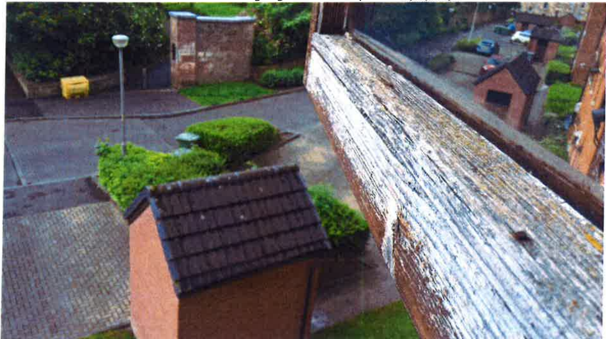
4. View of external timber bead and lack of appropriate sealant at junction with glazing.
