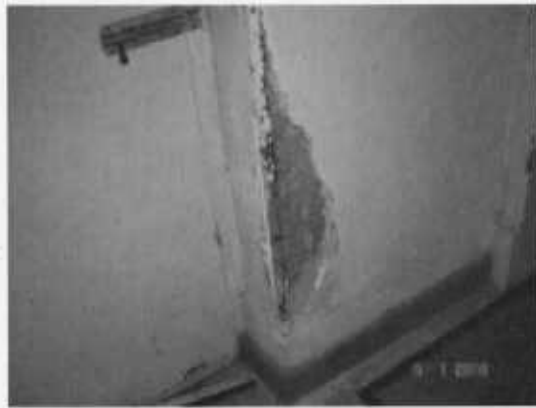
Defective plaster-rear door
