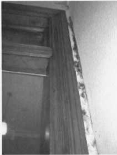
Mould at Hall door frame
