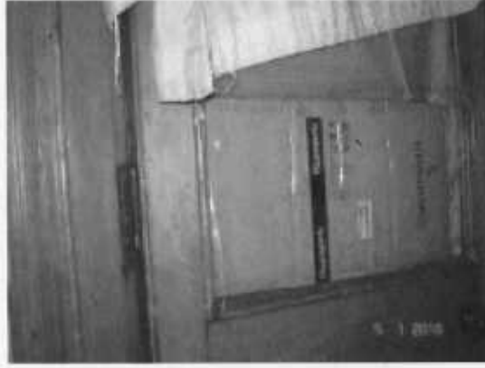
Broken glass – Hall door
