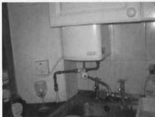
Water heater -Kit sink
