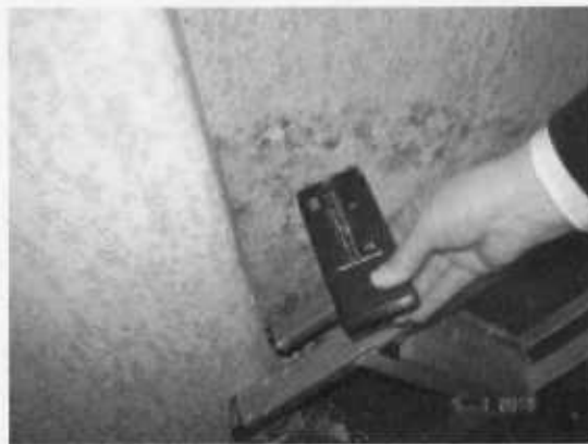
Damp readings adjacent to main door
