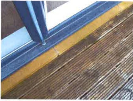
5. Ponding at screen external cill
