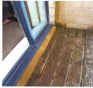
6. Ponding at screen external cill
