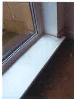
3. Screen – water damage at cill and skirting
