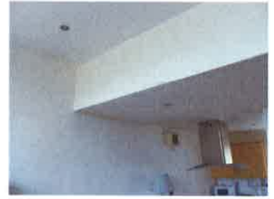
7. Water damaged kitchen ceiling
