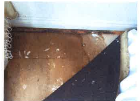
4. Screen – water damaged chipboard flooring and carpet
