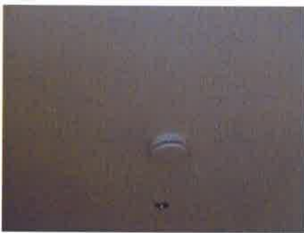
8. Hall smoke detector
