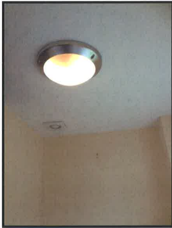
Figure 6 En-suite shower room extractor fan
