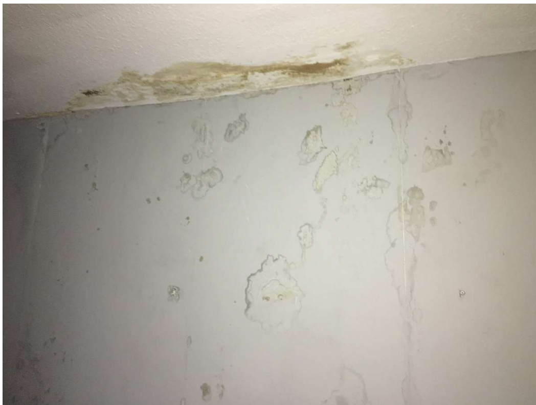
Damp staining to ceiling and north wall of NW Bedroom
