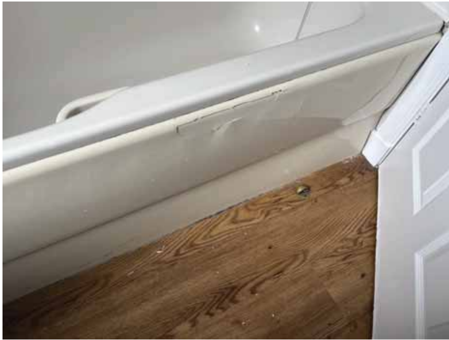
Cracked bath panel
