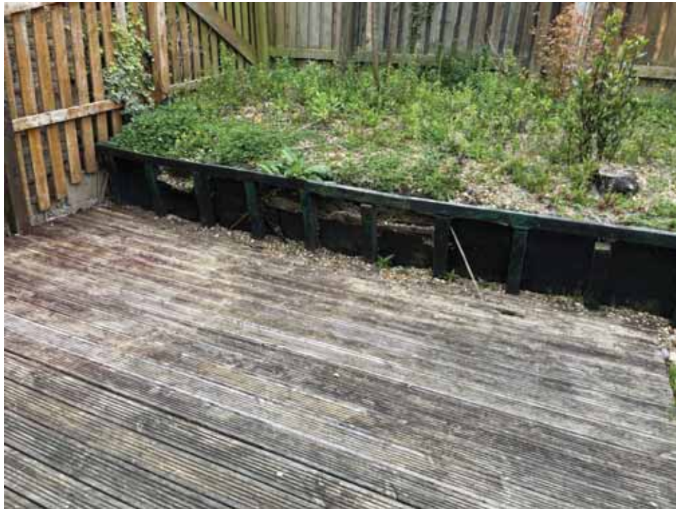
Failing retaining barrier
