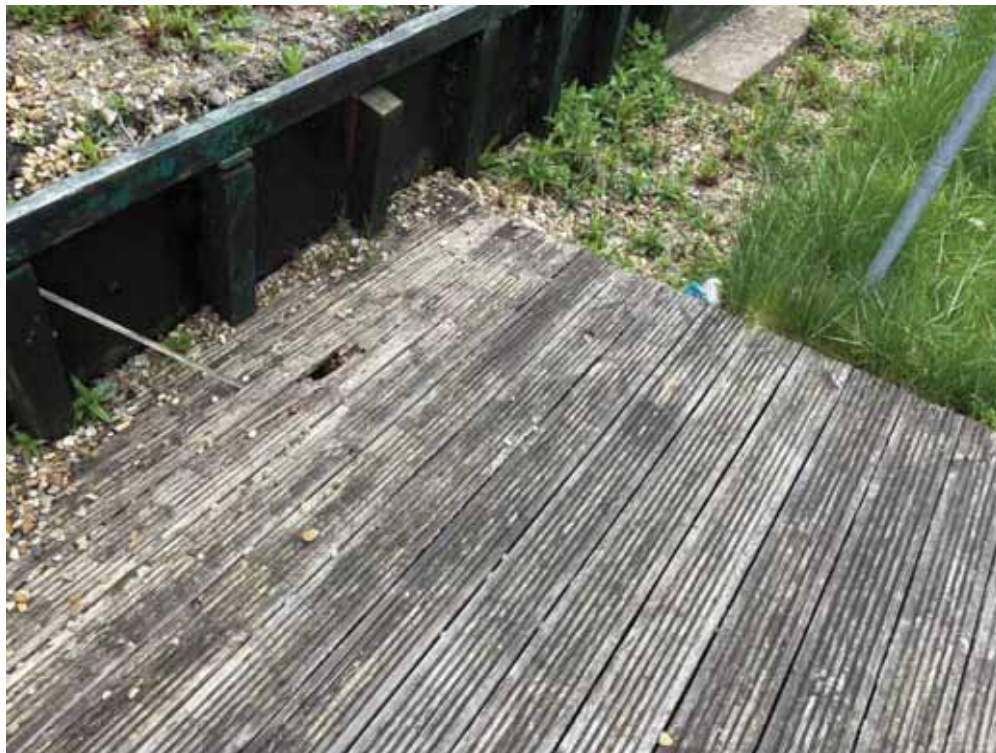
Small area of rot in decking
