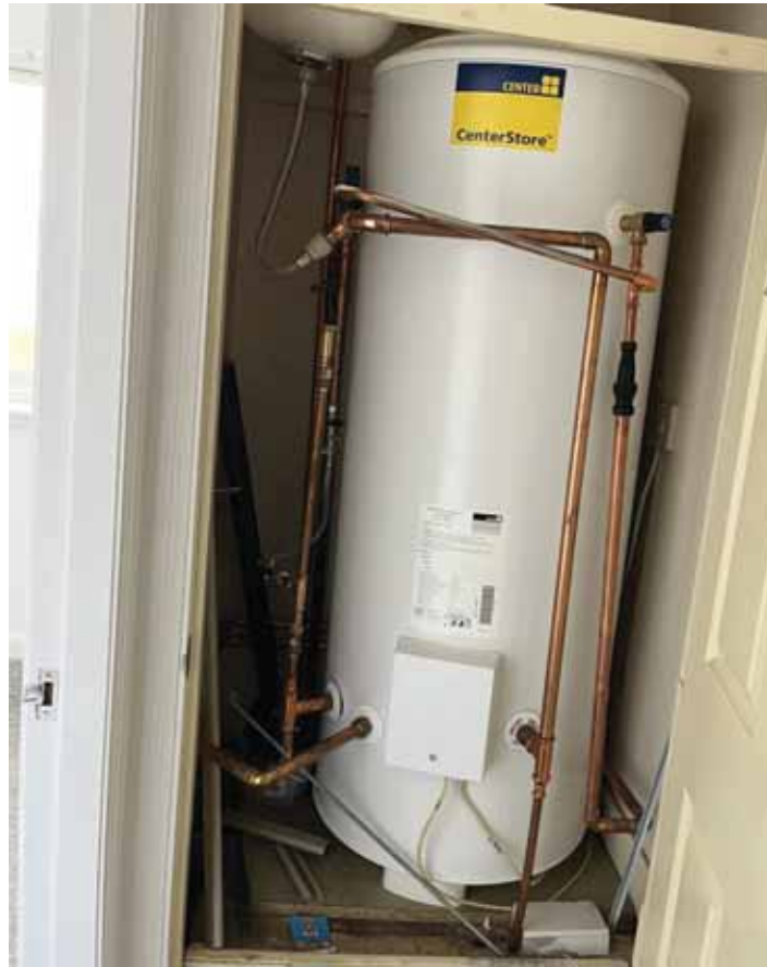
New hot water storage tank
