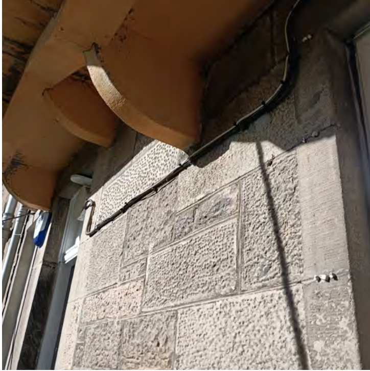
Photo 7: External mains cable
