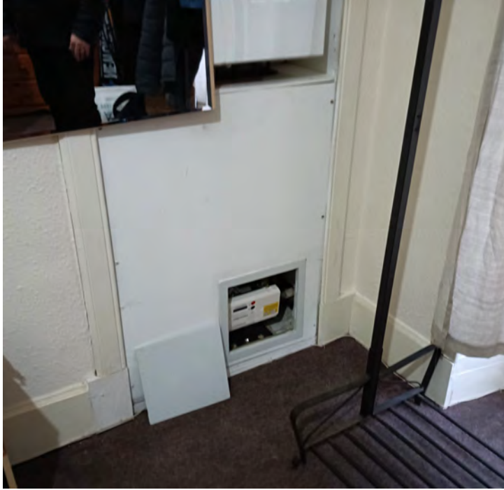
Photo 5 - Low level gas meter
