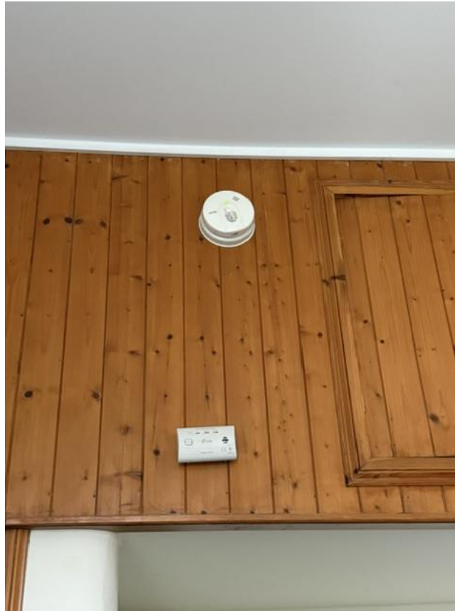
Photograph 6: Siting of heat detector and carbon monoxide detector to kitchen/dining area
