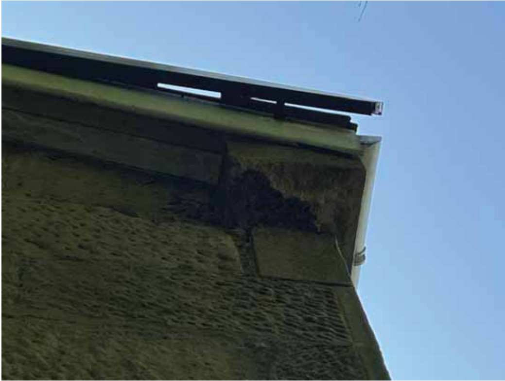
Loose roof verge
