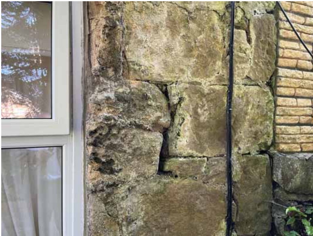
Missing mortar joints
