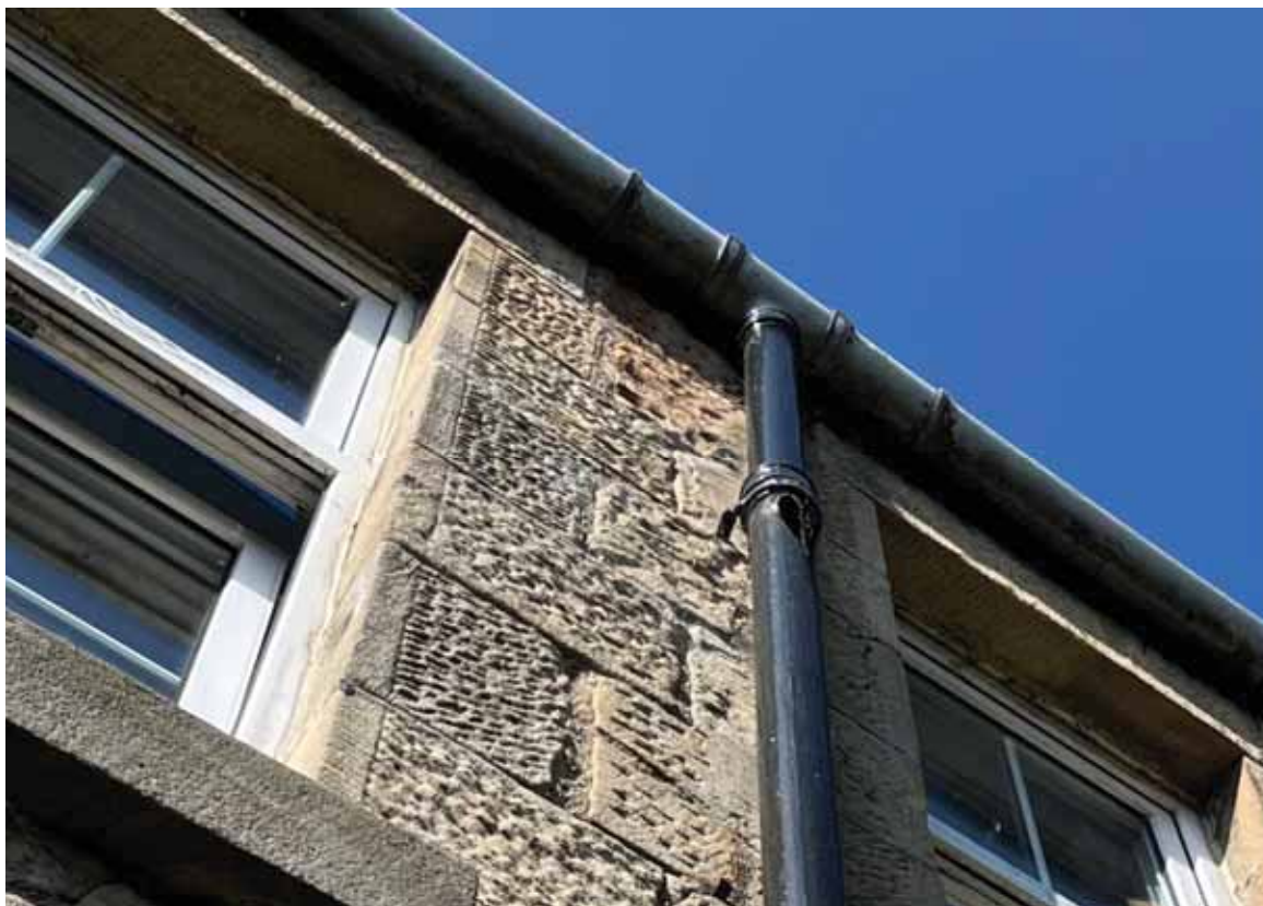
Hole in the downpipe
