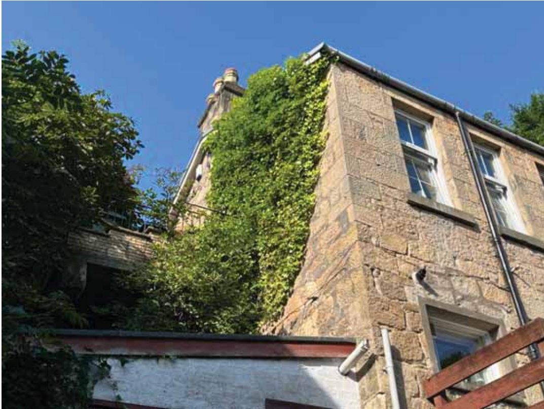
Climbing plant covering the wall and affecting the roof
