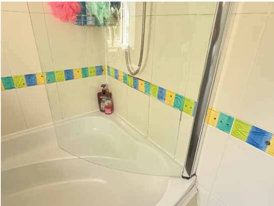
Loose wall tiles in the bathroom
