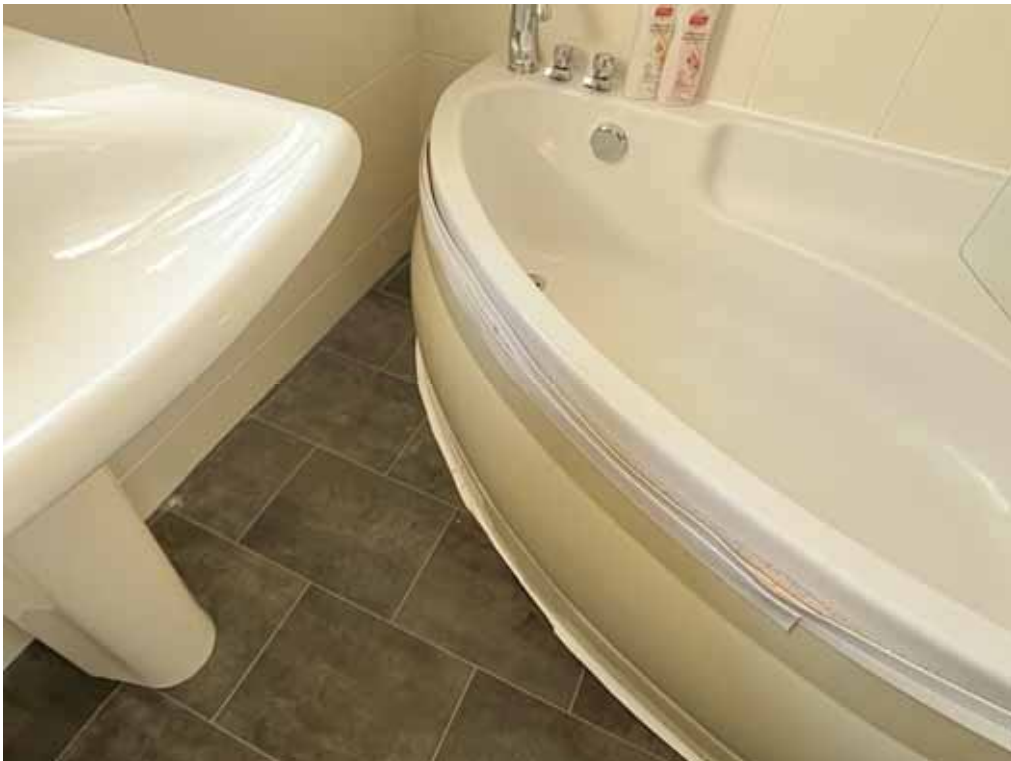
Loose bath panel
