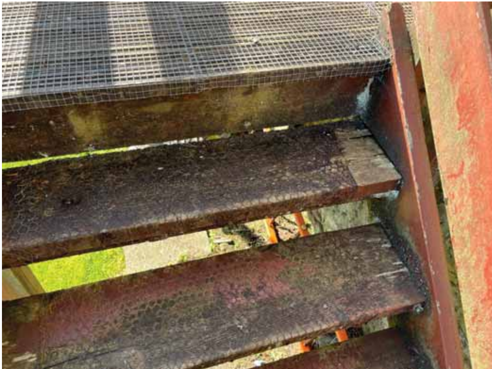
Loose top step
