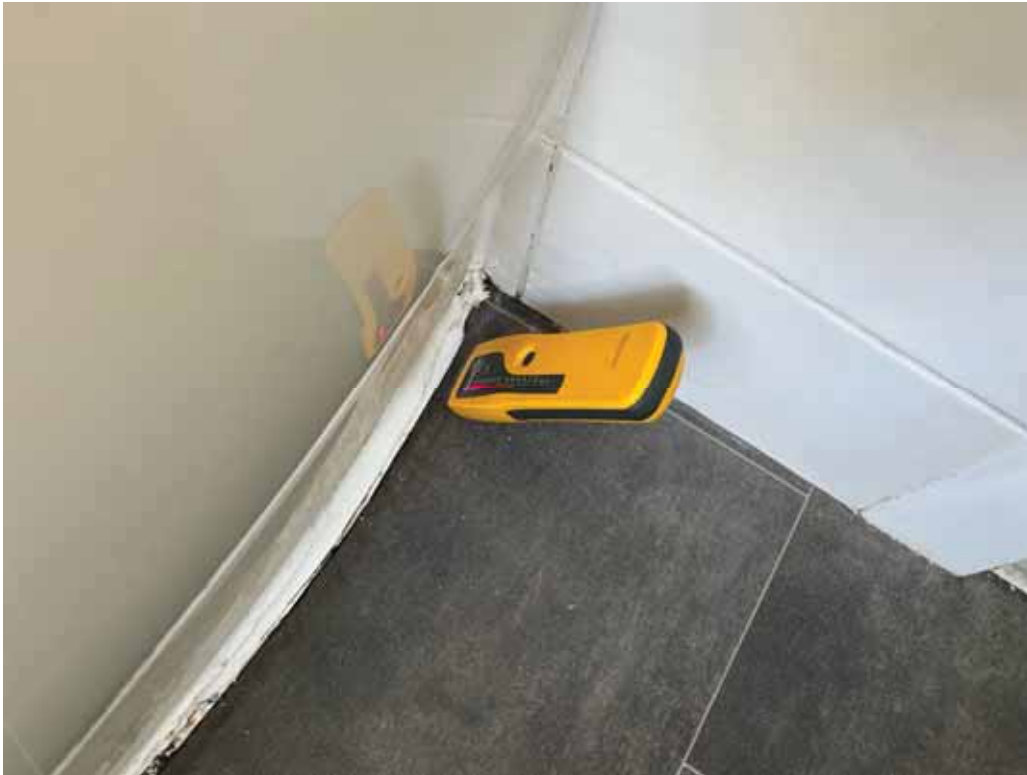
High moisture meter readings in the floor of the bathroom
