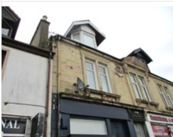
Front elevation - general deterioration to external building fabric
