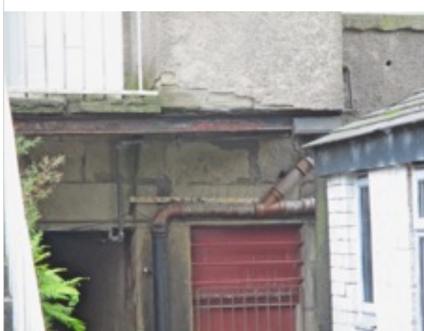
Rear elevation - roughcast spalling to wall on back projection adjacent to front door of flat 119a
