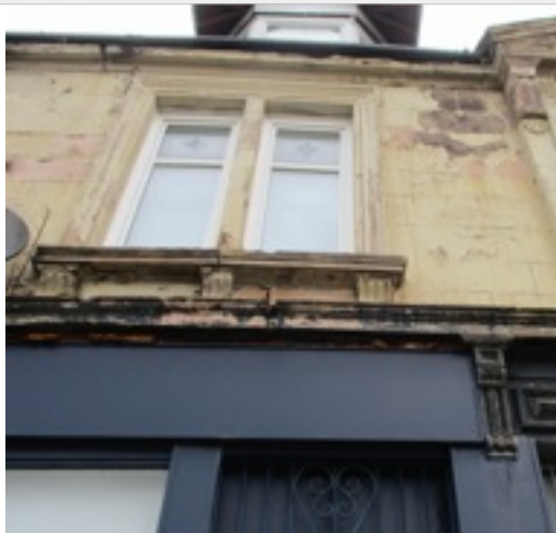
Front elevation - showing first floor window/ surrounding masonry - erosion to sill, cracks, water damage to upper stonework
