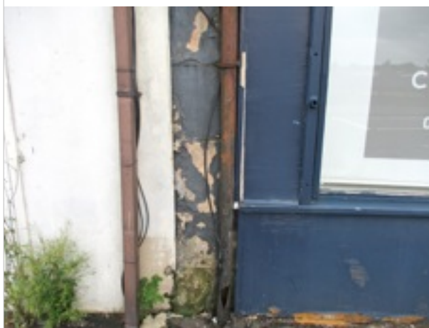
Front elevation - view of ground floor shop unit below subject property - paint peeling/exposed stonework and defective cast iron downpipe
