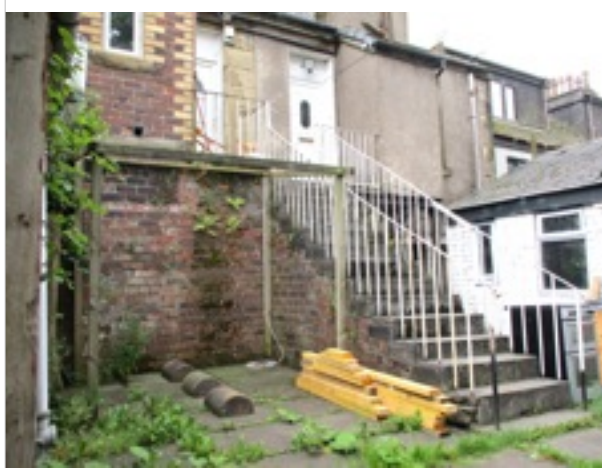
Rear elevation - showing common access steps and backcourt area - brickwork requires pointing, vegetation growth and bottom step damaged
