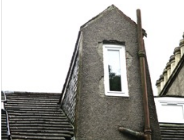
Rear elevation - roughcast spalling around dormer window
