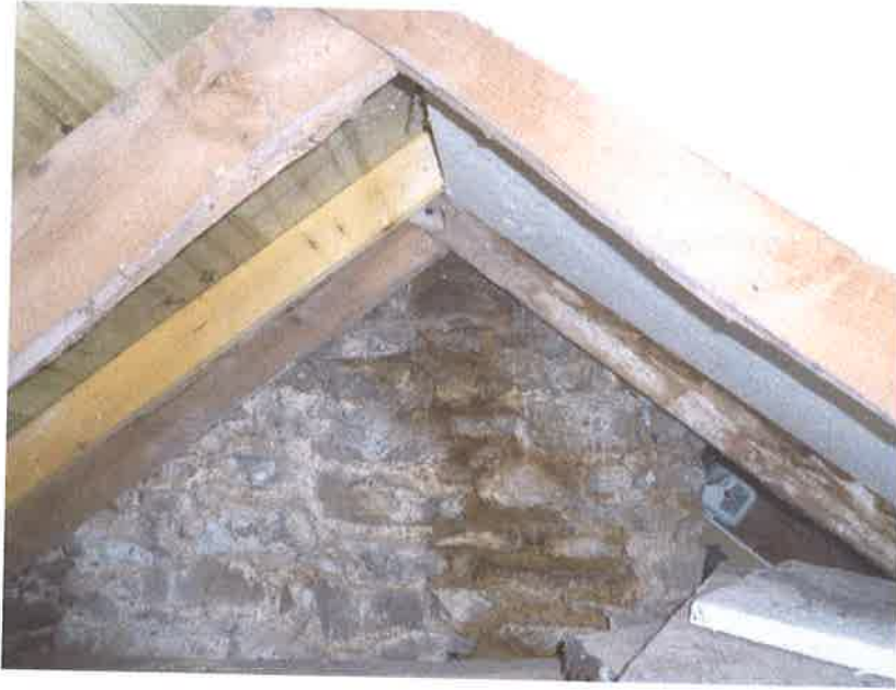
13. Cracking and water damage to chimney in roof space
