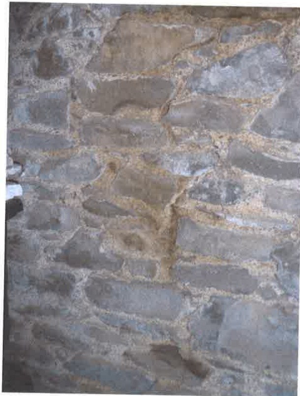
14. Cracking and water damage to chimney in roof space
