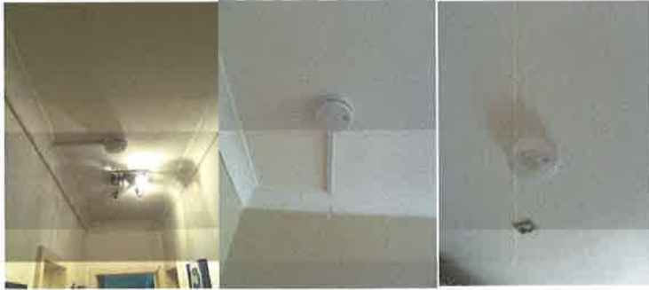
Fire Detection Equipment September 2016
