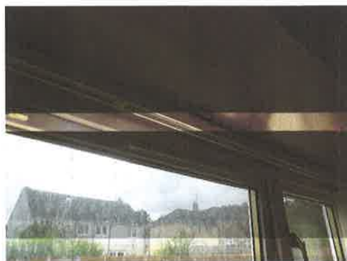
Trickle Vents at Windows - September 2016
