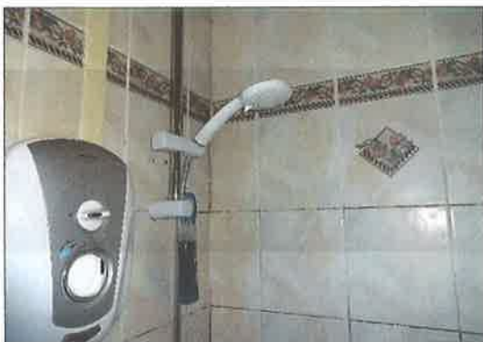
Loose shower head - Shower head replaced slight leak at seal
