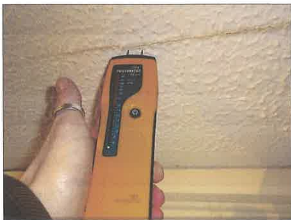
Wet patched hall ceiling – historic water marks no evidence of recent water ingress
