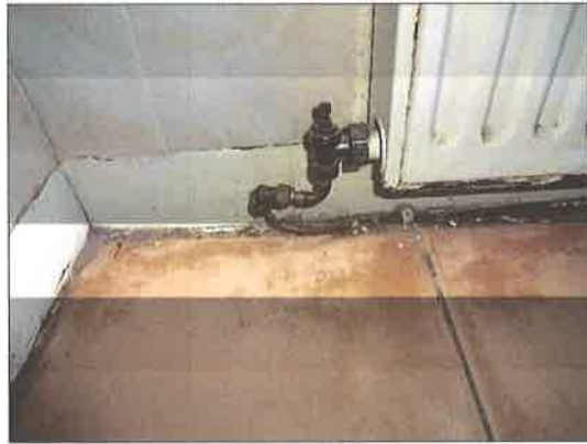
Mould/rot and leaking Radiator – Repaired
