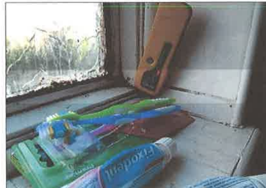
Mould within bathroom – Condensation
