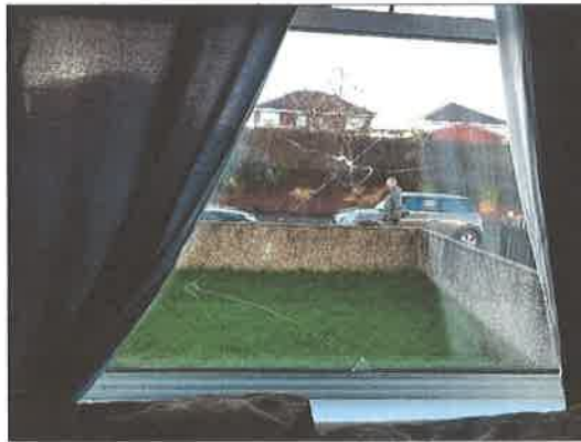
Broken living room window
