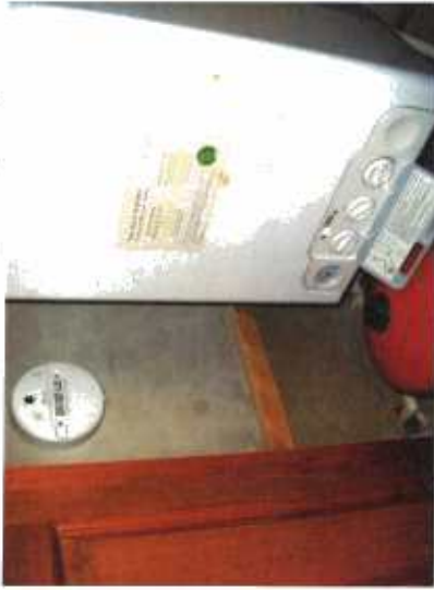
04 - Carbon monoxide alarm at boiler
