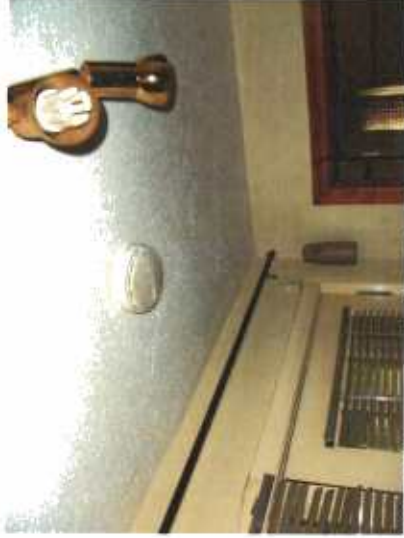
02 - Battery-operated smoke alarm, lower hall
