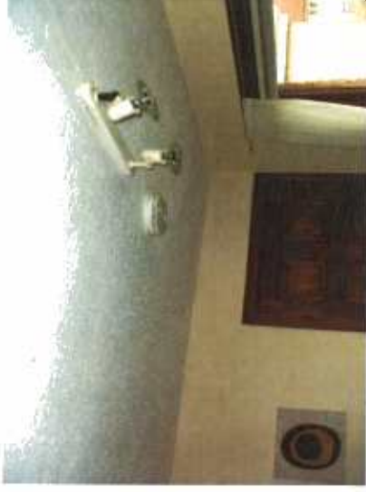
03 - Battery-operated smoke alarm, upper hall
