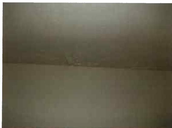
08 - Upstairs bedroom - dampness on NW gable
