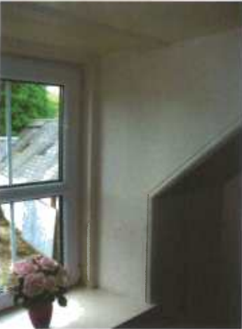
13 - Dampness at dormer haffit
