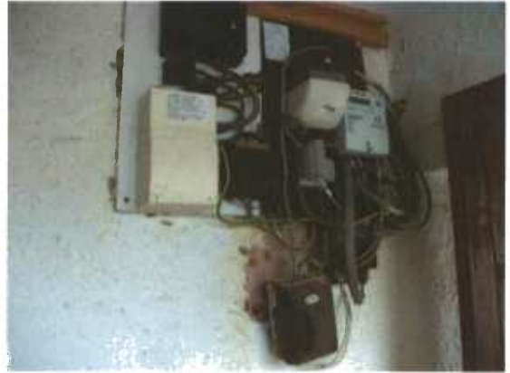
12 - Main electrics board at inspection
