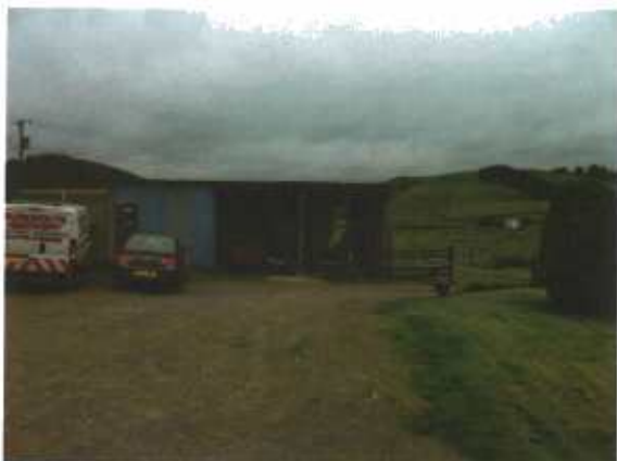
05 - Shed (wood store) with missing sheeting
