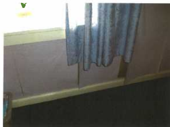
06 - GF bedroom - loose wallpaper
