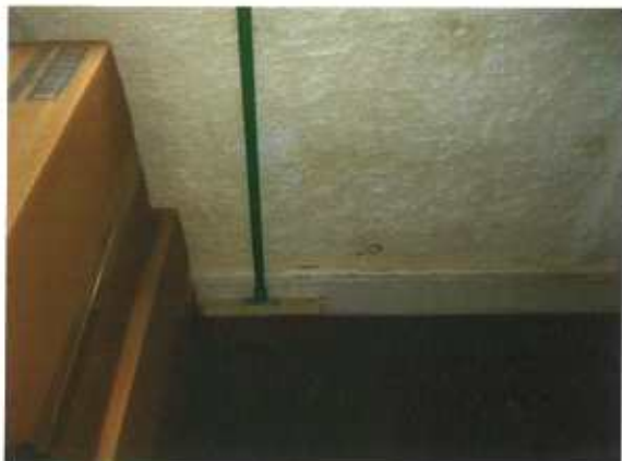
07 - Rear porch - dampness and defect
