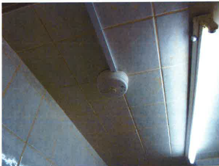
2. New heat detector - kitchen.
