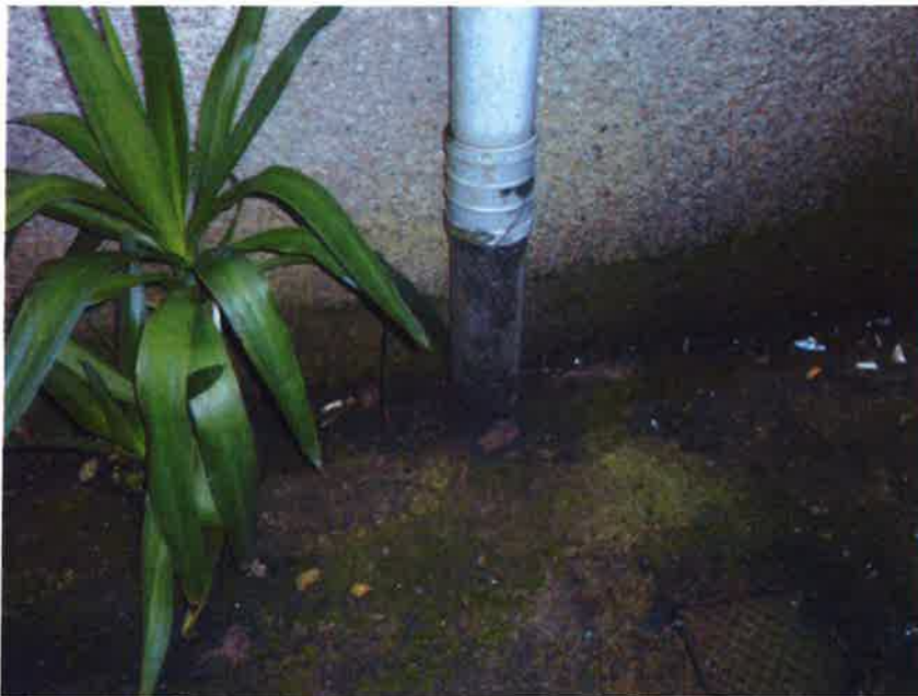
4. Defective down pipe to rear
