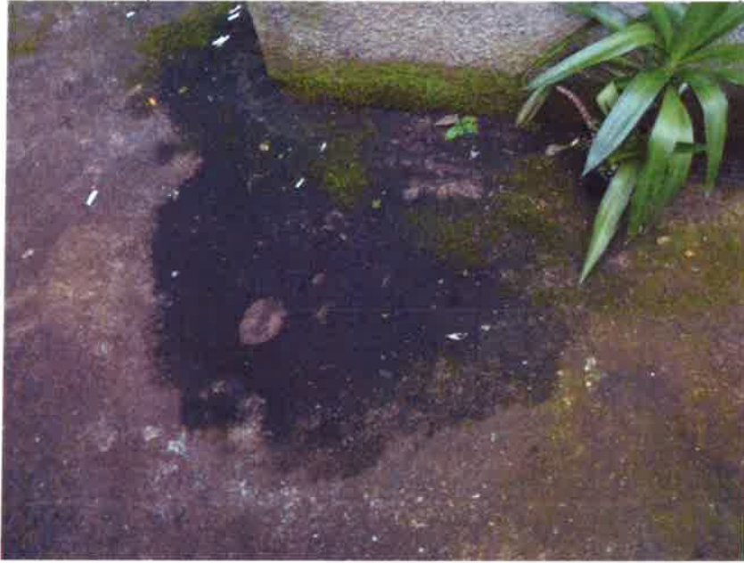
5. Area of ponding adjacent defective downpipe
