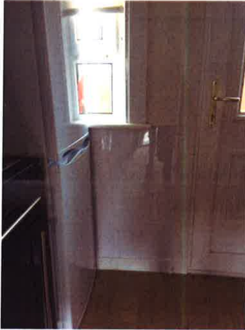
Previously damp wall in kitchen next to back door
