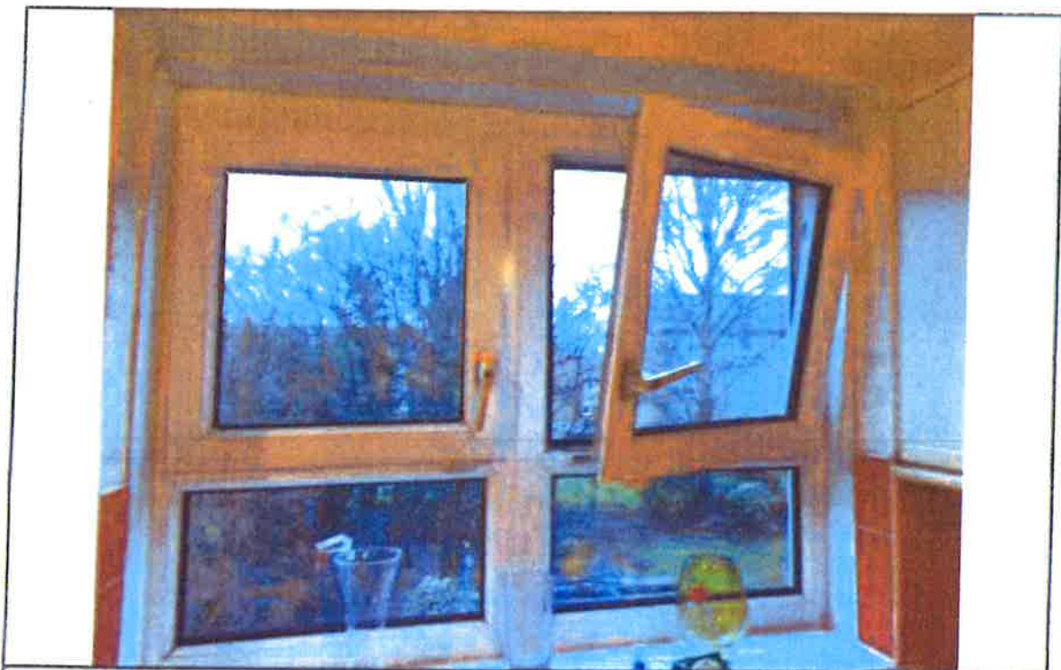
1. Kitchen Window 24 January 2017
