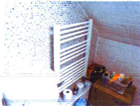
Shower room Radiator 3 rd April 2017
