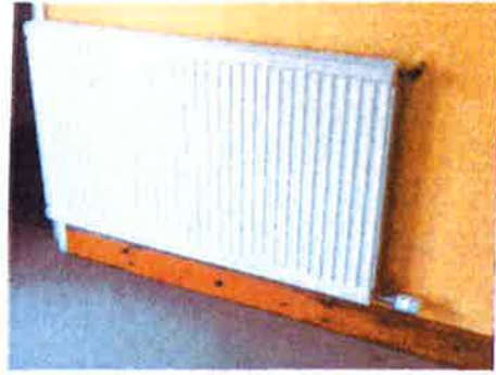
Dining Room Radiator 19 th June 2017
