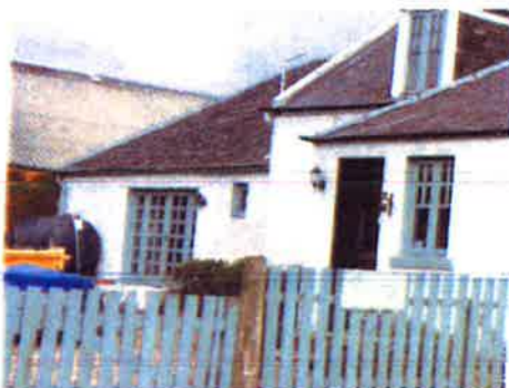
No external soil stack vent 3 rd April 2017
