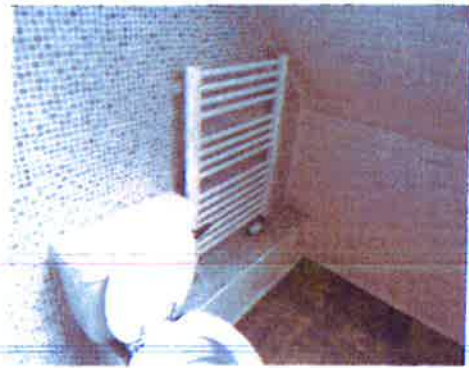
Shower Room Radiator 19 th June 2017
