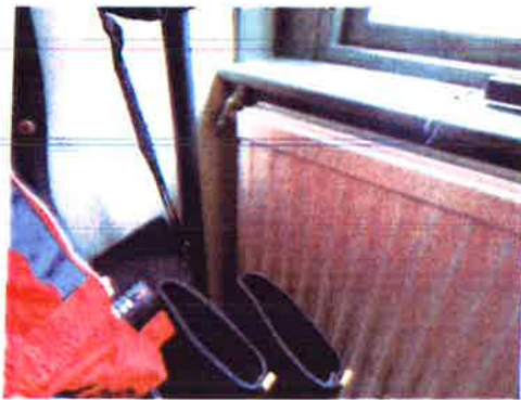
Hall Radiator 3 rd April 2017
