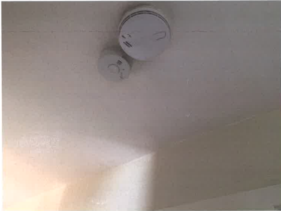
Smoke detection system in hall
