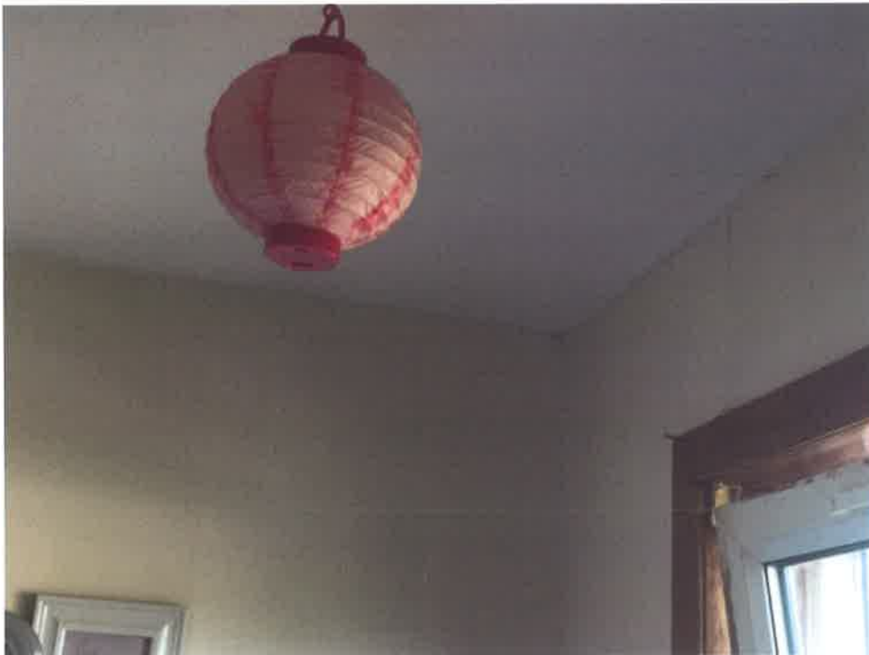
Bedroom 2 – north – reduced damp staining in corner
