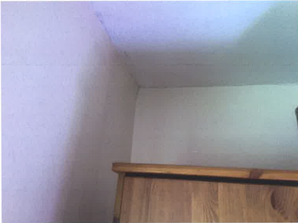
Bedroom 1 – south – reduced damp staining in corner
