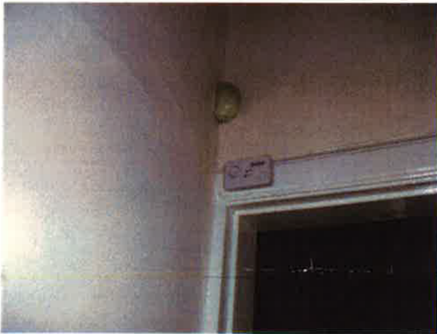
03 - Kitchen - carbon monoxide detector
