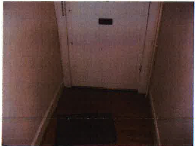
04 - Main entrance door - draught-excluder fitted
