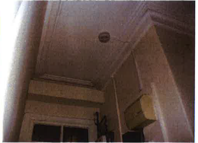
02 - Hall - hard-wired smoke detector
