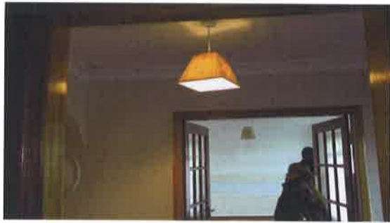
Photo 2 – Functioning hallway light fitting
