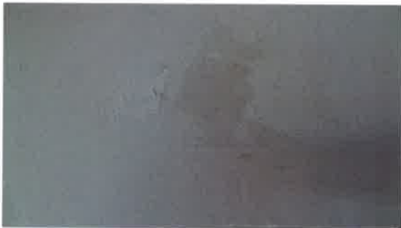
Photo 4 – Former Lounge wall light location
