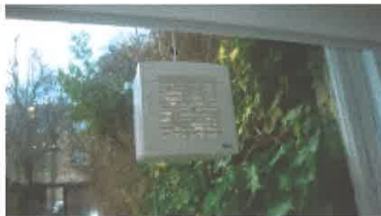
New electric ventilator in kitchen
