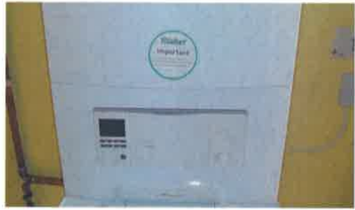
Photo 7 – Replacement gas boiler
