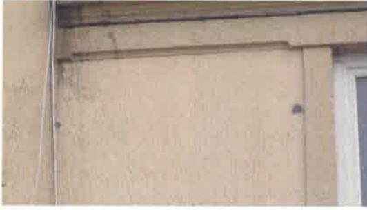
Photo 6 – Patched holes on front elevation
