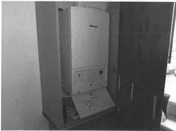
3:- Gas combination boiler
