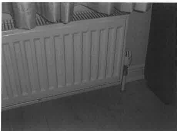
6:- Living room radiator & thermostatic valve
