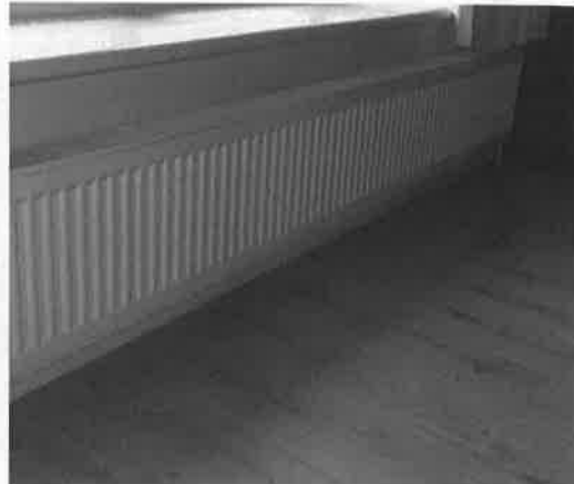
7:- Living room radiator
