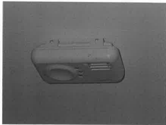
4:- CO detector on kitchen ceiling
