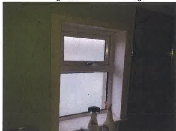
4 Bathroom – no trickle ventilation of extract ventilation.
