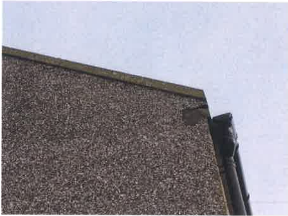
15 Cracking to gable elevation at high level.
