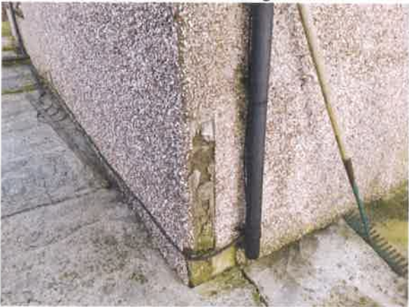
17 Section of damaged render.
