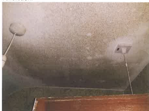
6 General mould growth within Bathroom.
