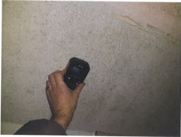
7 Elevated moisture readings within Bathroom.
