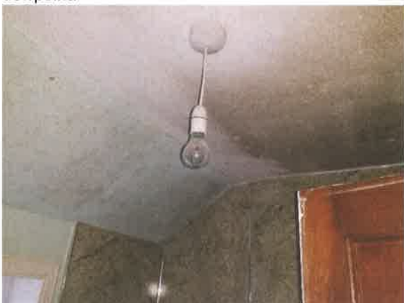
5 General mould growth within Bathroom.
