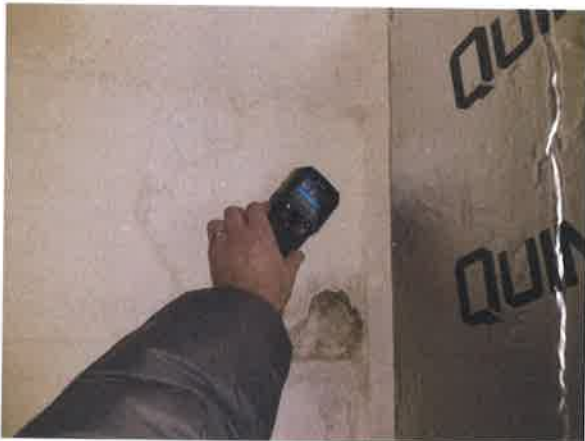
9 Area of elevated moisture readings within Bedroom.
