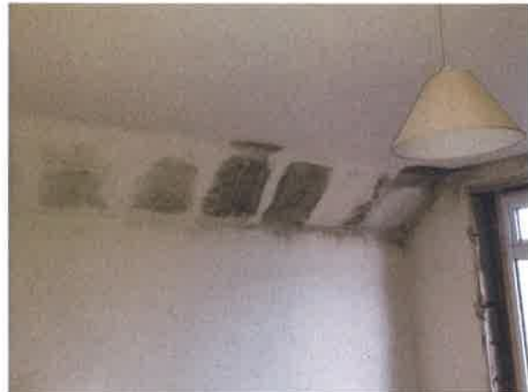
2 View of mould growth to coombed ceiling.
