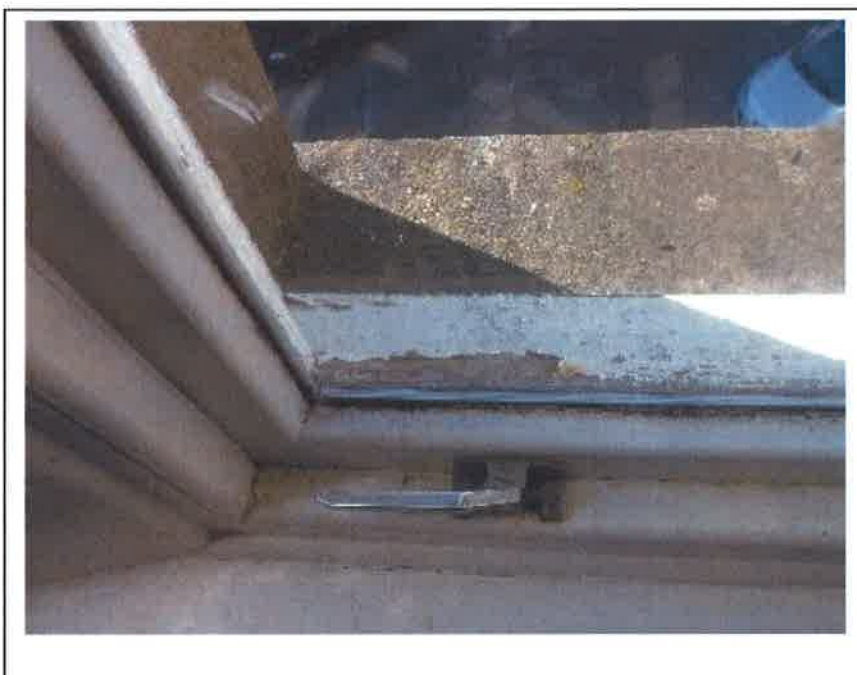
Weathered windows require ongoing maintenance
