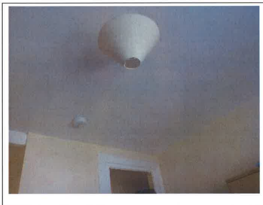
Historic damp staining within kitchen, tested dry with damp meter at inspection.
