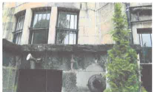
Photo 13 Rotten/missing fascia board
