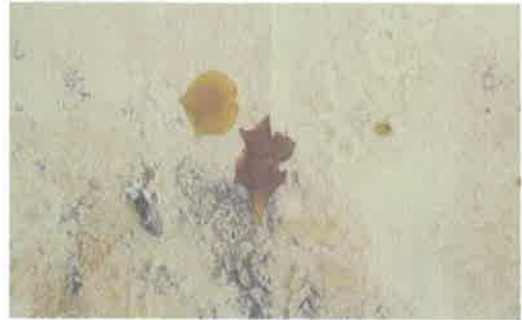
Photo 3 Fungal growth in Living room
