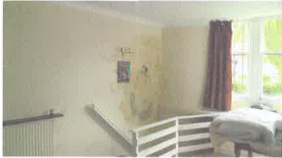
Photo 2 Water damage in Living room (L/R)
