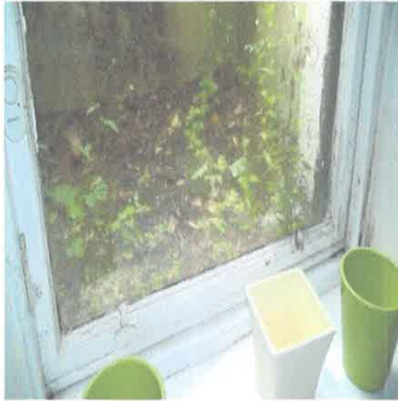
Photo 14 Severe damp at front bed. window
