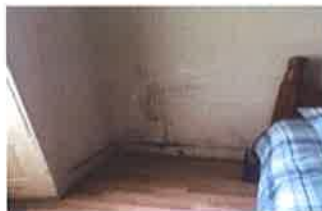
Photo 3 – Bedroom dampness and rot
