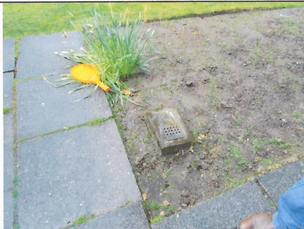
6. Cover at head of drain in rear garden
