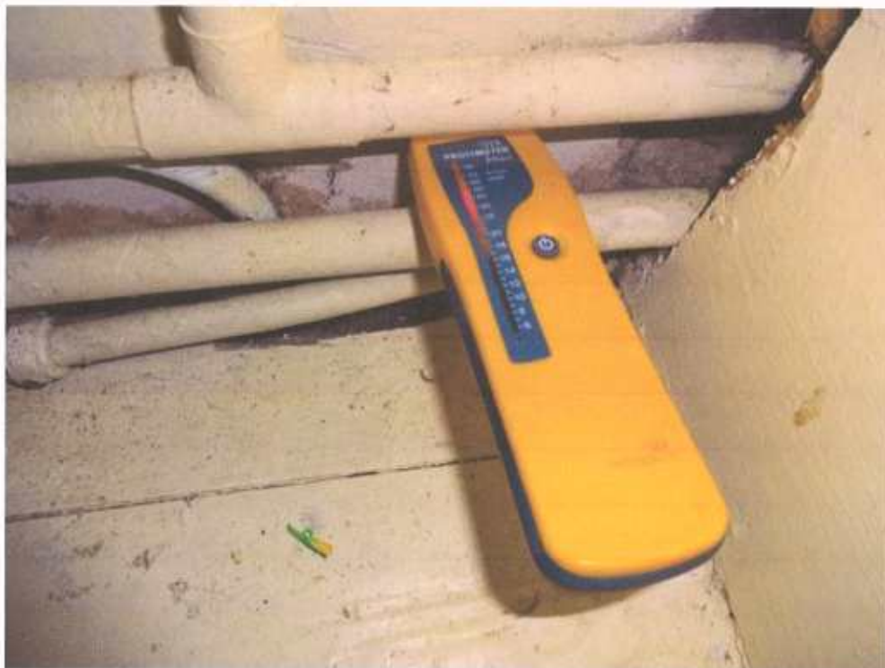
Kitchen cupboard reading 60% +moisture recorded
