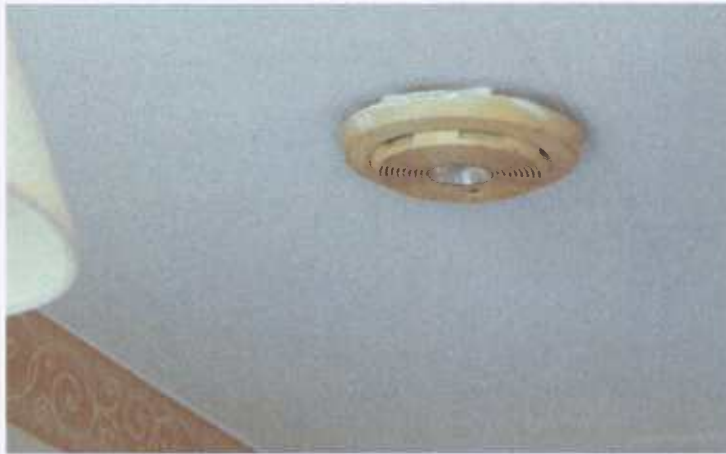
Photograph 1 :- Battery operated smoke detector in Hall.
