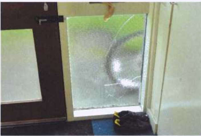
Photograph 5 :- Cracked glass panel at entry door.
