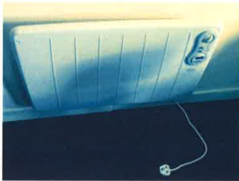
Electric panel heater – living room 20 June 2016
