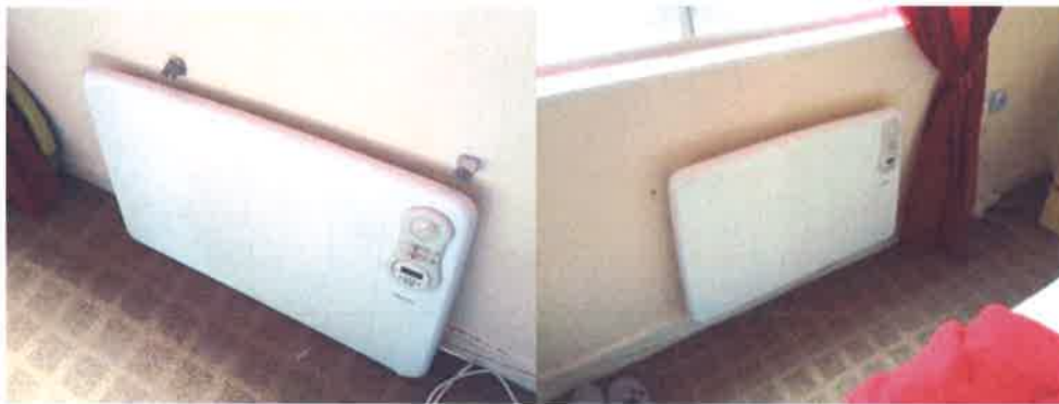
Electric panel heater – bedroom 20 June 2016
