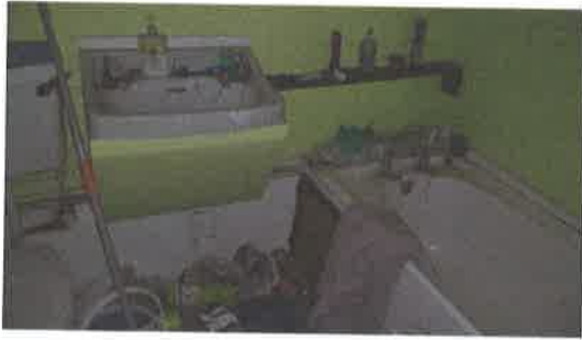
Photo 8 – Bathroom in poor condition
