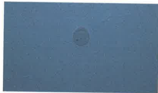
Photo 11 – Batt. operated alarm in L/R
