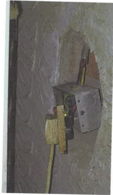
Photo 3 – Unsafe cooker connection
