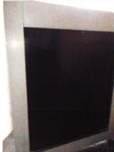
Kitchen - lower section of external door, panel missing to internal side
