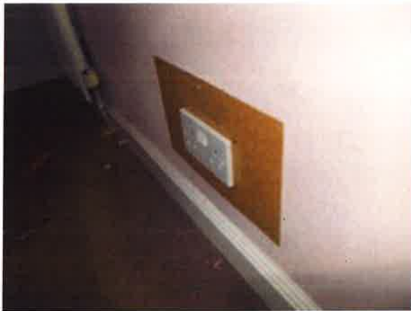
Bedroom (3) to rear - double socket replaced and surrounding hole covered by tenant
