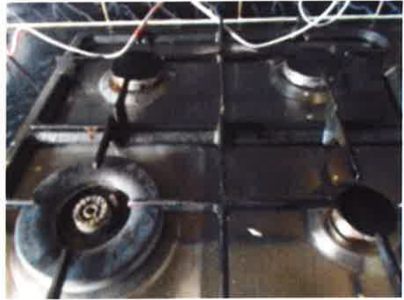
Kitchen - Gas Hob - One gas burner cap missing
