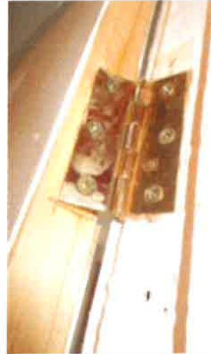
Bedroom (2) to front - Door hinges defective/loose screws
