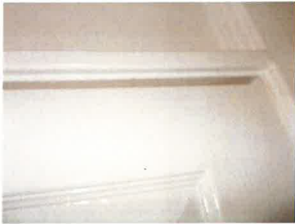
Bedroom (2) to front - Ill fitting door - gap at top
