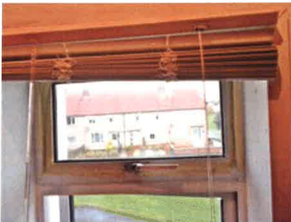
Landing - Window - top light taped shut
