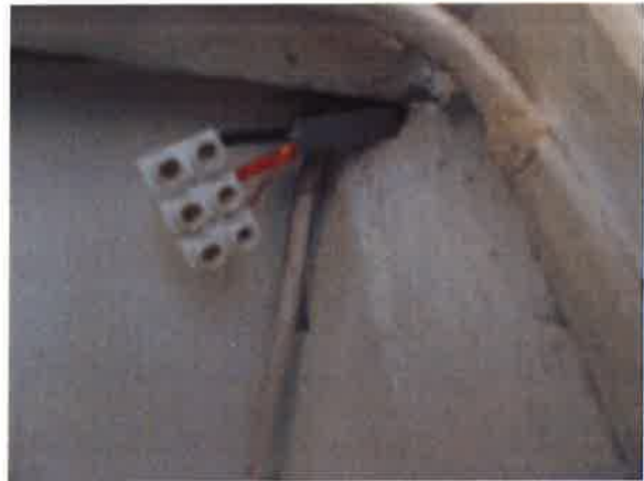
Ground Floor hall cupboard under stairs - exposed wires capped with a terminal block
