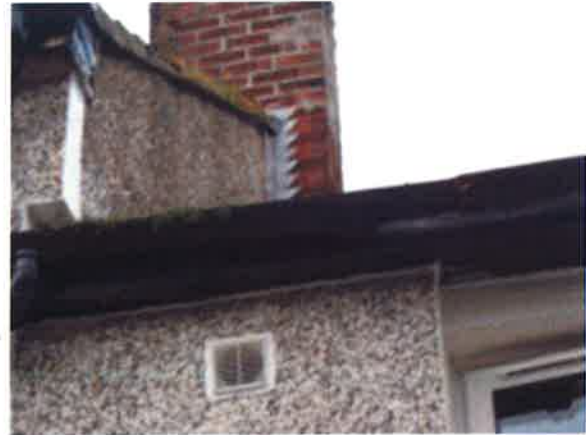
Front Elevation - gutter choked with vegetation/ leaking and sagging
