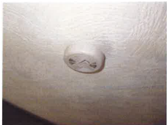
Ground Floor Hall - Ceiling mounted smoke alarm
