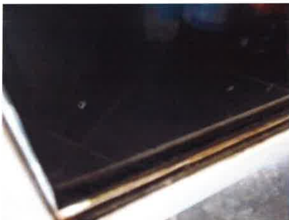
Kitchen - lower section of external door, panel missing to internal side
