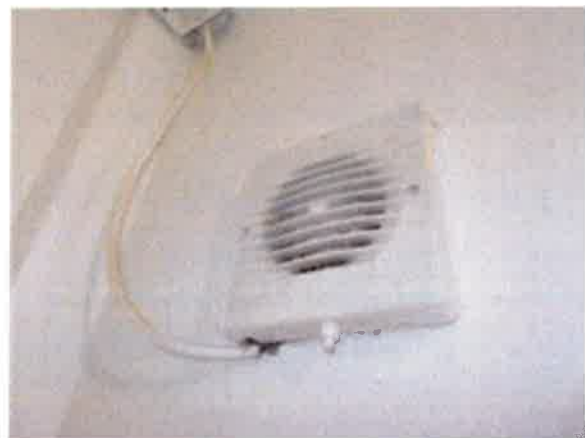
Bathroom - extractor fan, not fixed properly to wall/exposed wires
