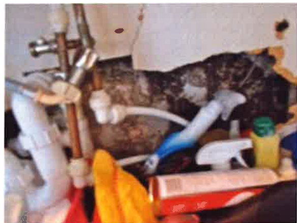
Kitchen - severe black spot mould to base of rear external wall under kitchen sink
