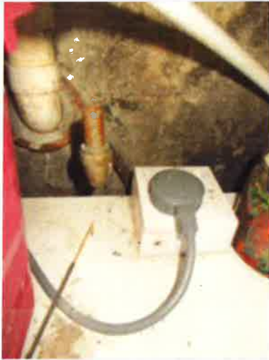
Kitchen - Single socket - located under sink (Observation)
