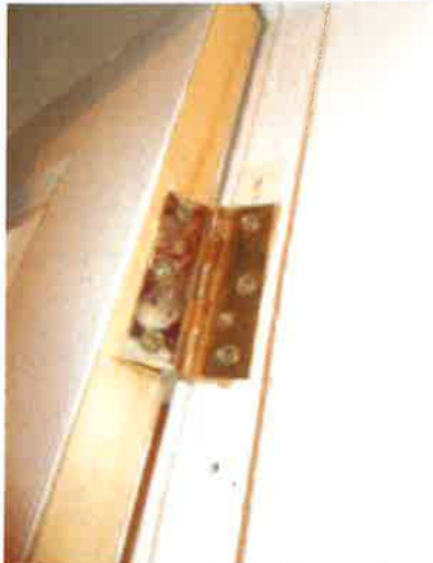
Bedroom (2) to front - Door hinges defective/loose screws
