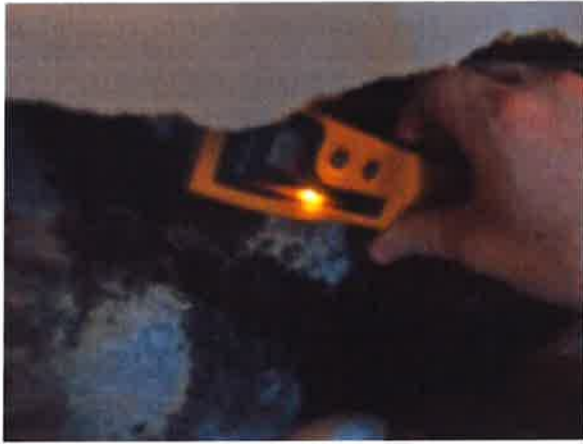
Kitchen - severe black spot mould to base of rear external wall under kitchen sink - amber damp meter reading (search mode)
