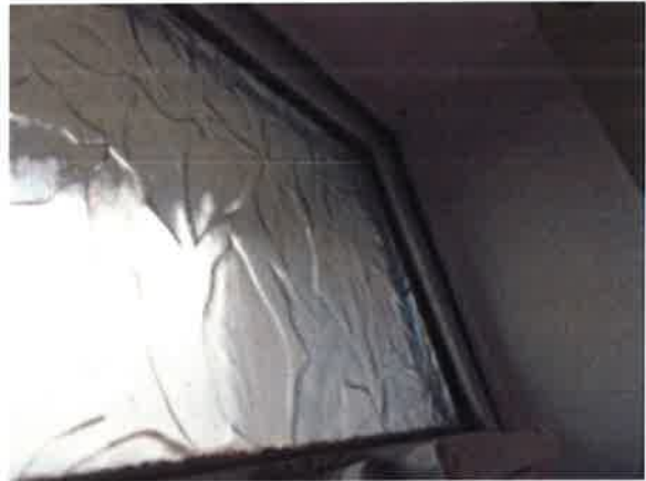
Bathroom - Window - top light wide gap at seals when closed from inside
