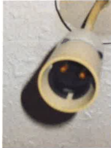
Bedroom (2) to front - defective central ceiling mounted light fitting
