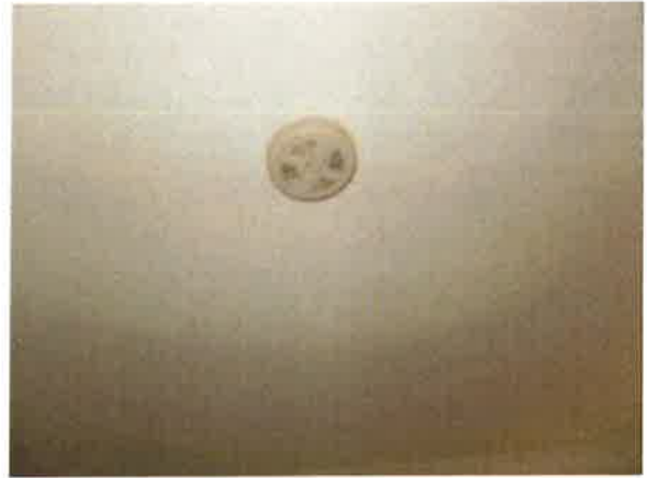
Living Room - Ceiling mounted smoke alarm
