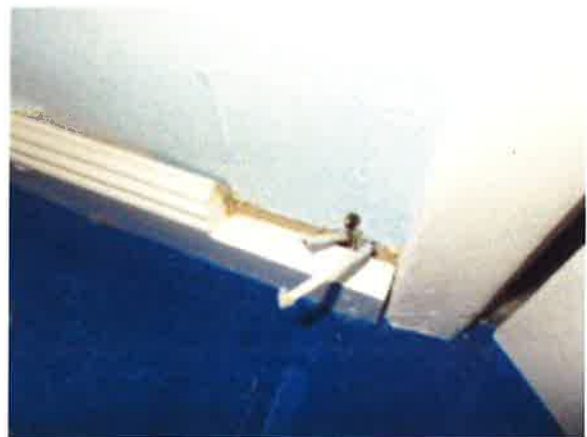
Bedroom (1) to rear - exposed wires above skirting board
