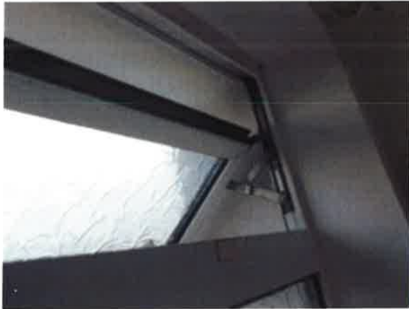
Bathroom - Window - top light defective mechanisms/does not open/close properly
