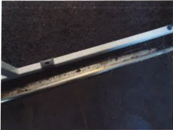
Living Room/Kitchen - exposed carpet gripper/ missing threshold bar
