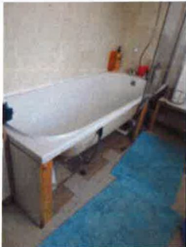
Bathroom - side bath panel missing
