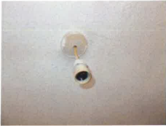
Bedroom (2) to front - defective central ceiling mounted light fitting
