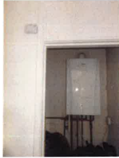
Bedroom (2) to front - Boiler housed in cupboard - new wall mounted CO alarm to left of cupboard door
