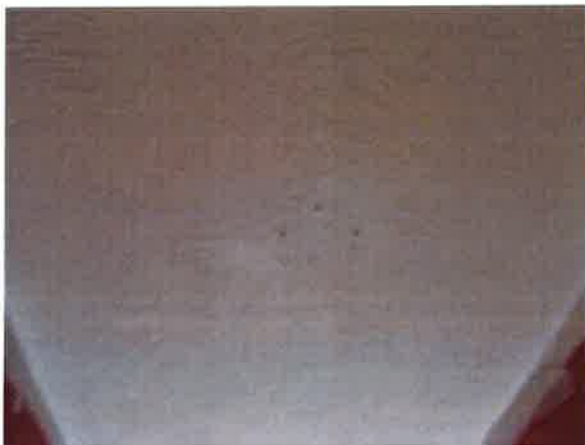
Upper Floor Landing - possible site of former smoke alarm - removed
