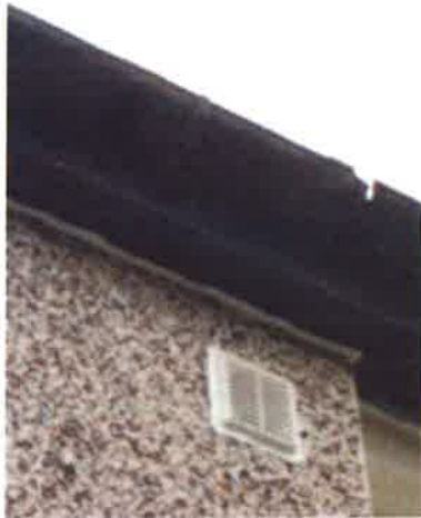
Rear Elevation - gutter broken/leaks at joints
