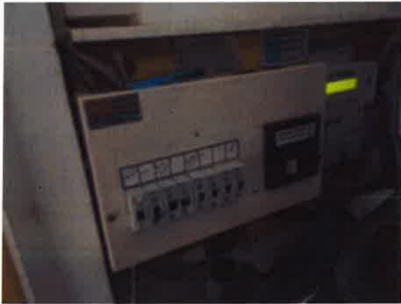
Ground Floor hall cupboard under stairs - Electrical Consumer Unit
