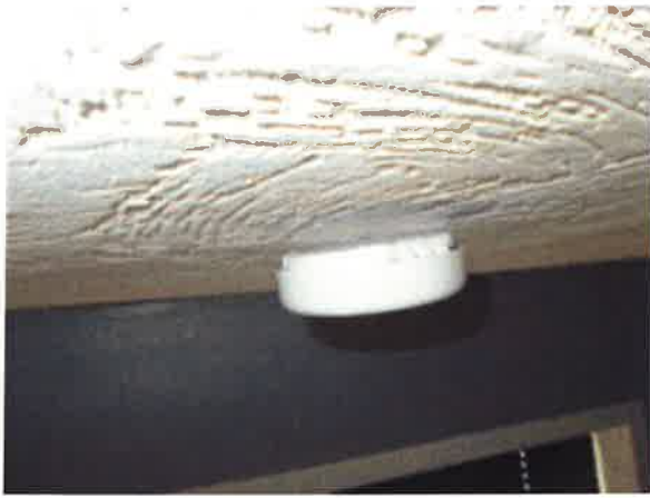
Ground Floor Hall - Ceiling mounted smoke alarm - not fixed properly
