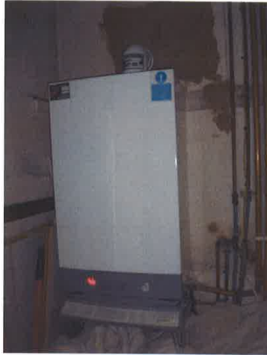
9. Gas central heating boiler
