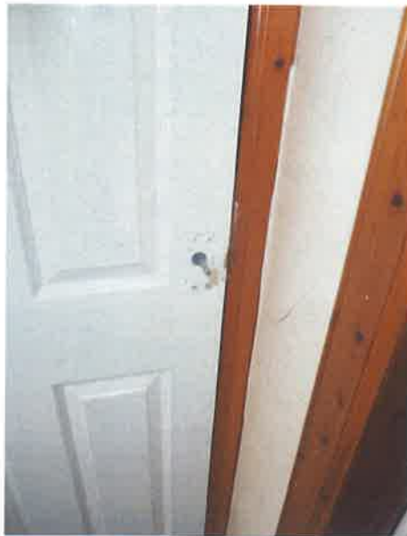
8. Handle missing from Boiler Cupboard door
