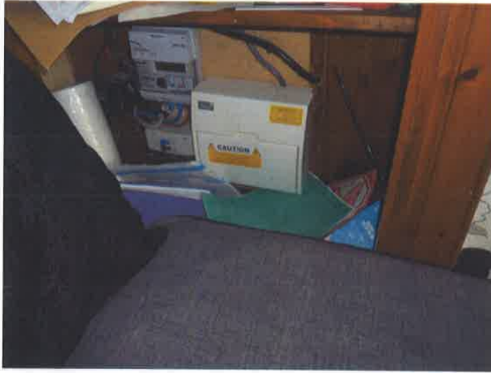
17. Electrical distribution board and meter
