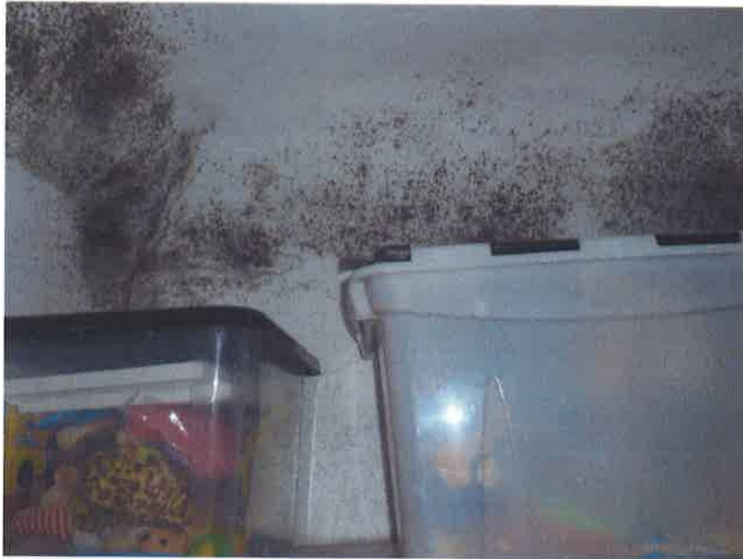
11. Mould in Front Bedroom cupboard
