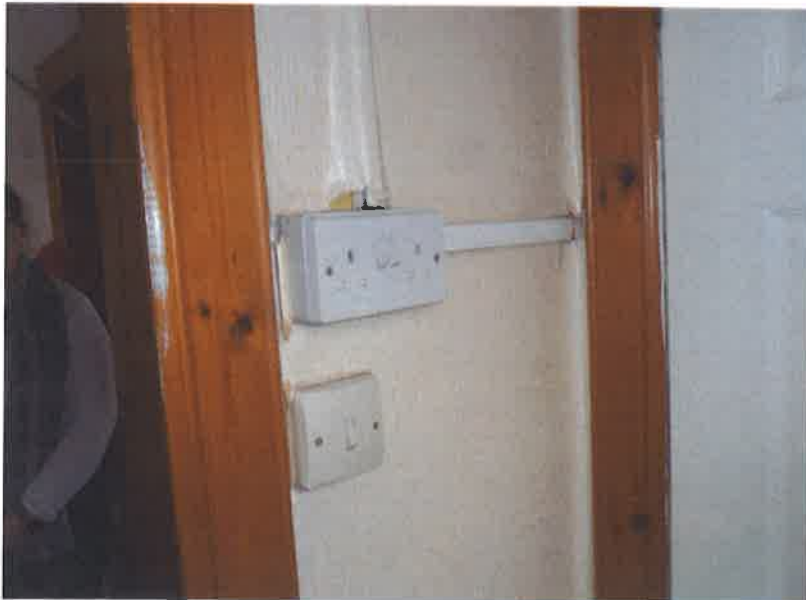
6. Loose double socket in vestibule
