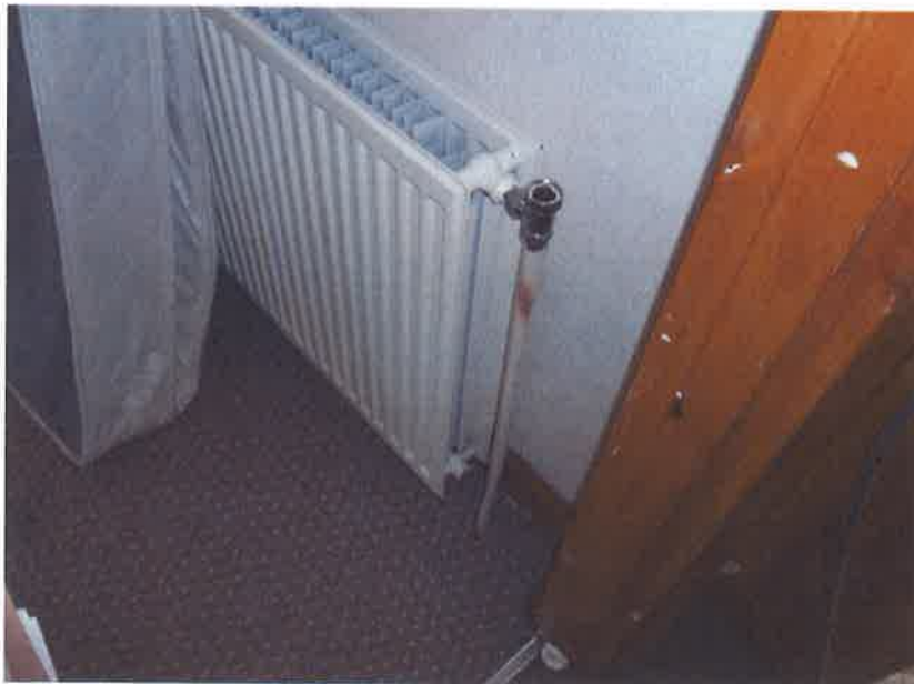
12. Missing radiator valve in Front Bedroom
