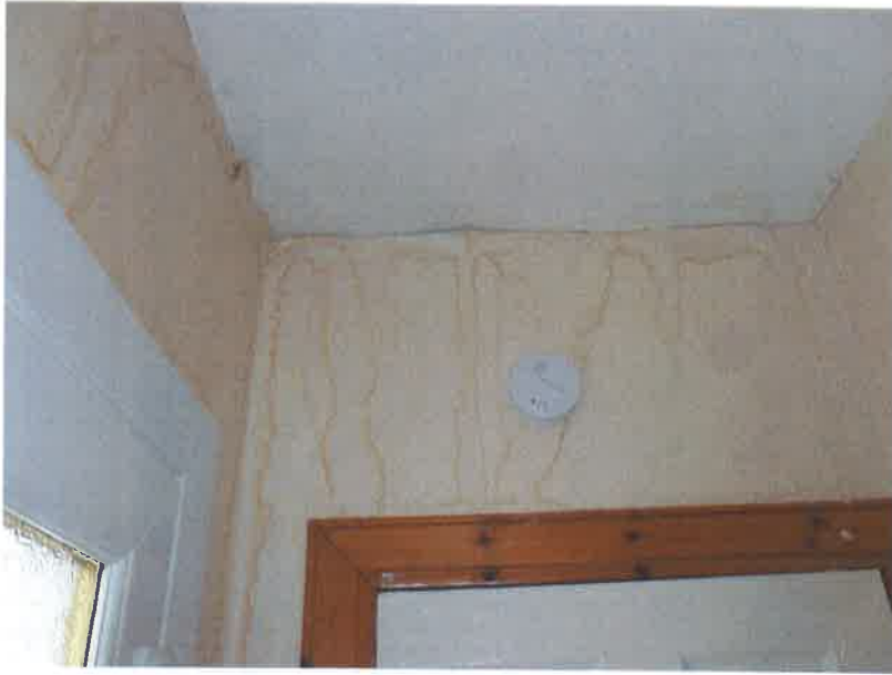
5. Water staining and carbon monoxide detector in Vestibule
