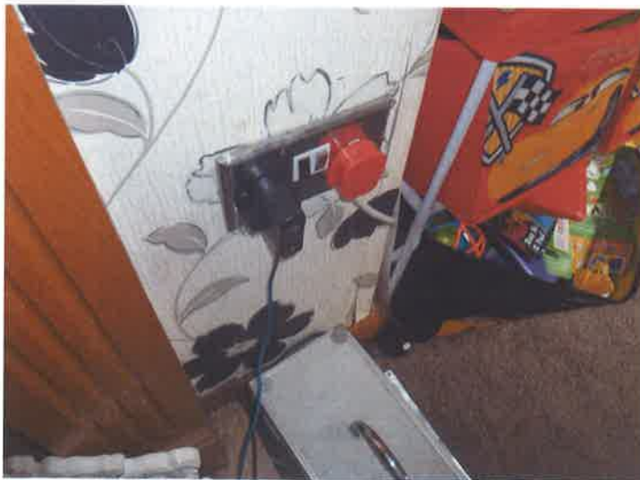
18. Defective socket in Living Room
