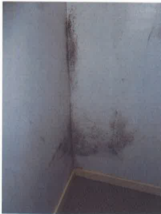
10. Mould in Front Bedroom cupboard
