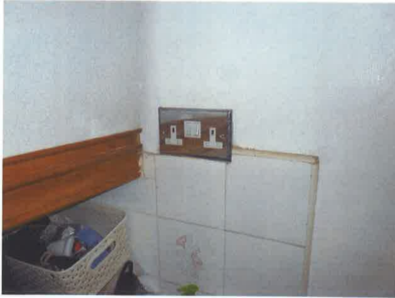
7. Defective double socket in Kitchen
