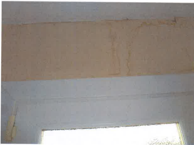
4. Water staining in Vestibule
