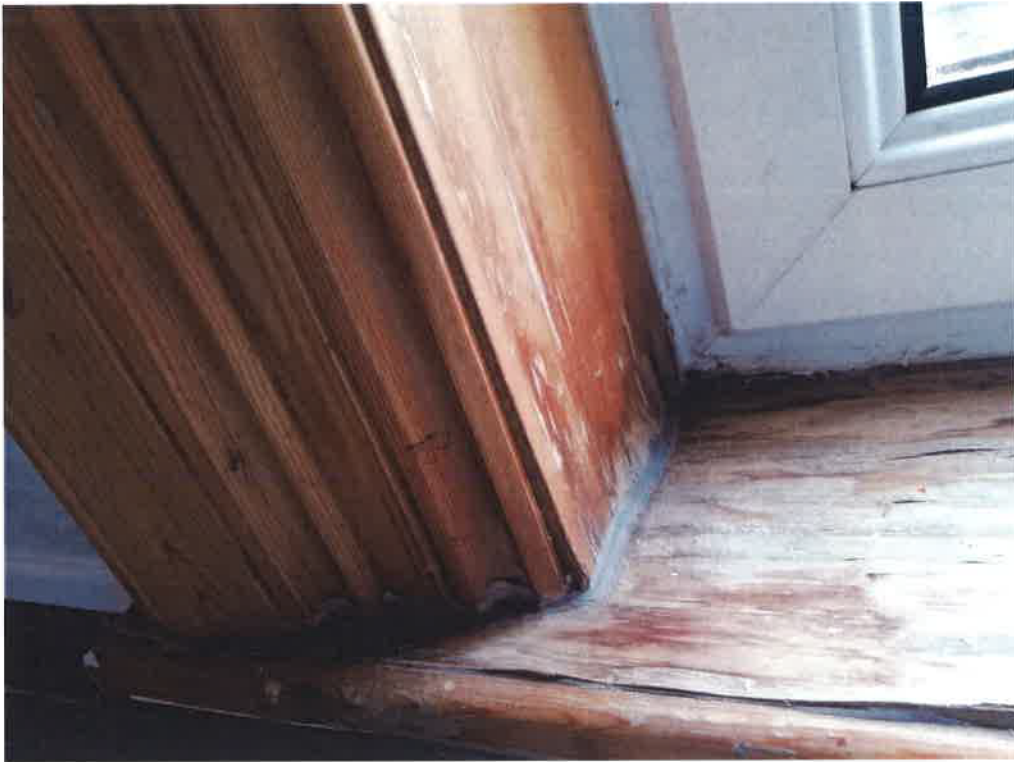
1R Potential dry rot in kitchen windowsill 2
