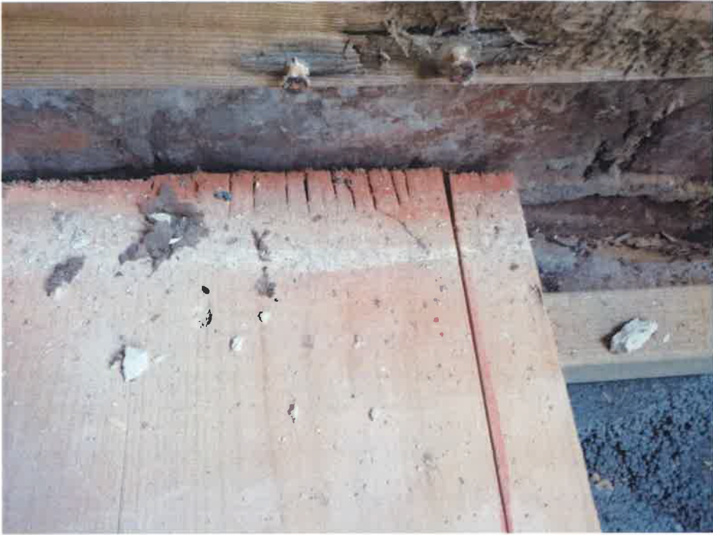
2R dry rot in floorboards
