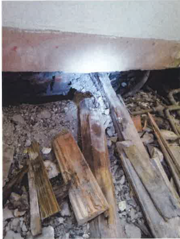
2R dry rot joist 1
