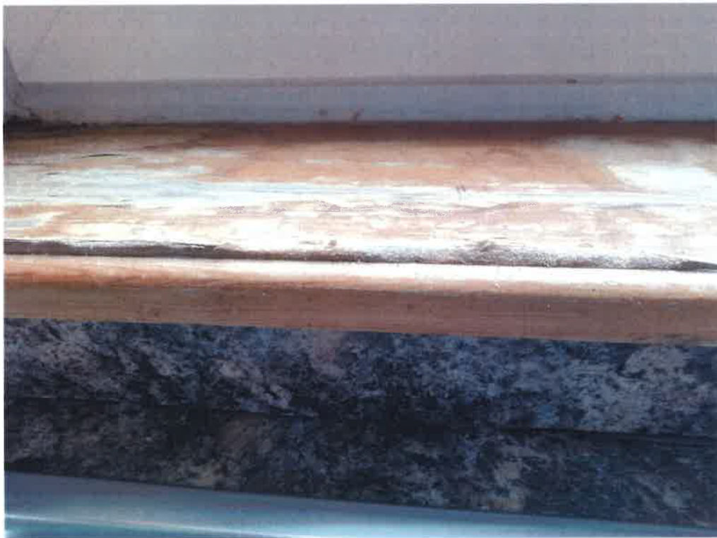
1R Potential dry rot in kitchen windowsill 1
