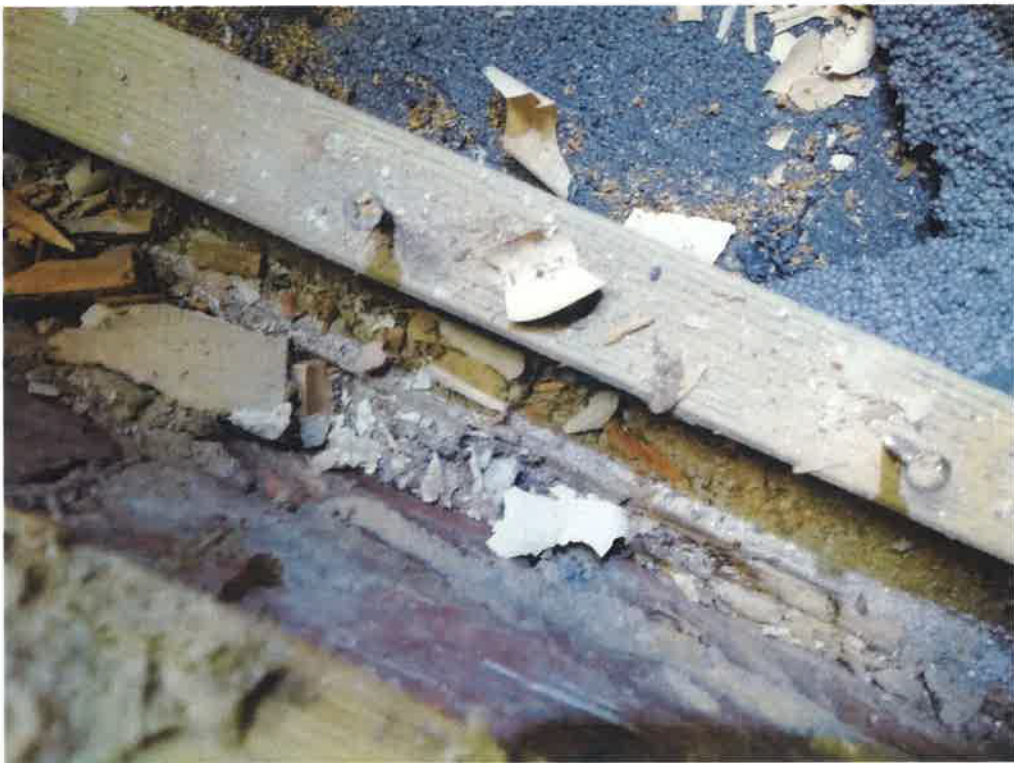
2R dry rot joist 2
