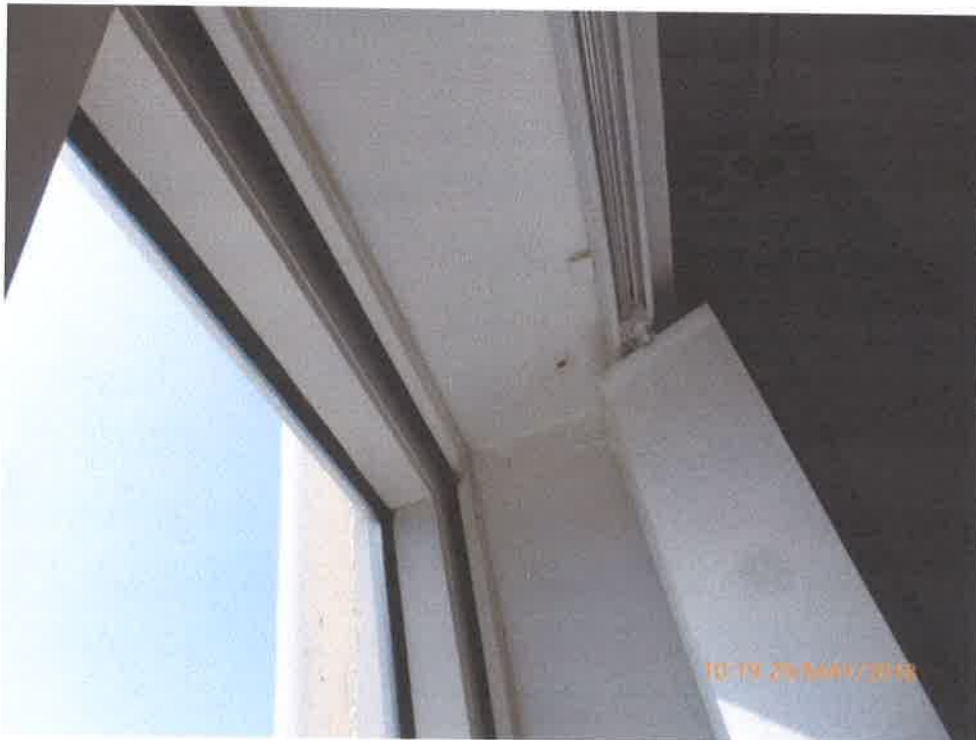
Detail showing gap in frame
