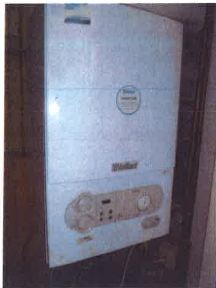
8. Gas central heating boiler.
