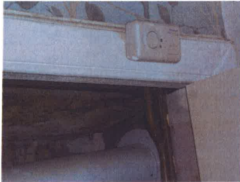
9. Carbon monoxide detector in living room
