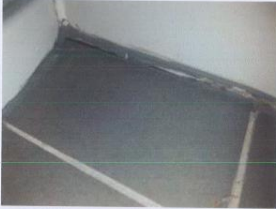
1 Gap opening up at junction between floor tiles and sealant.
