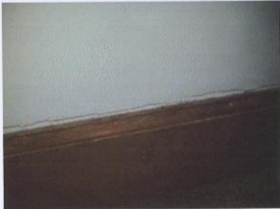
7 Hairline cracking at skirting.
