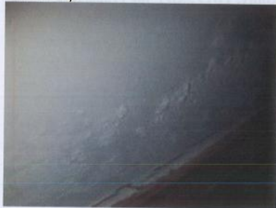
6 Close view of wall adjoining shower and water damage.
