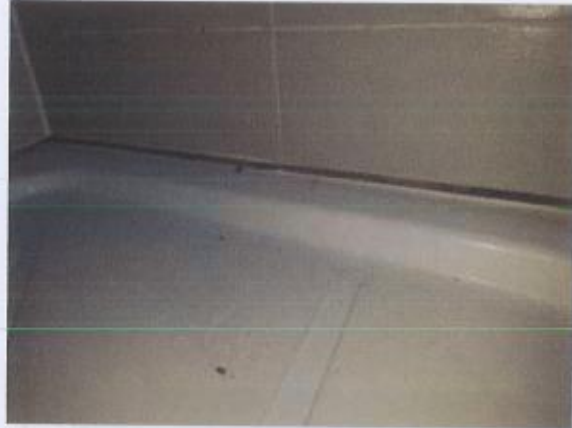
2 Noticeable gap at junction with shower tray.
