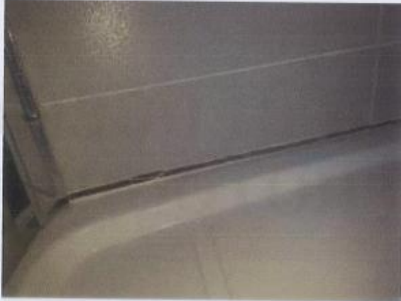
3 Further view of noticeable deflection at shower tray.
