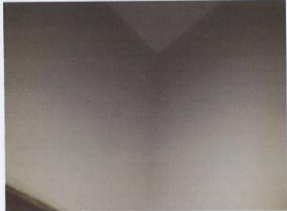
8 Vertical hairline cracking at corner.
