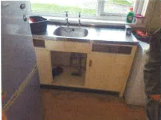
19 Missing components of kitchen base unit.
