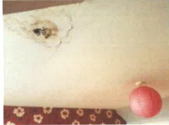
26 Water damage within Bedroom.
