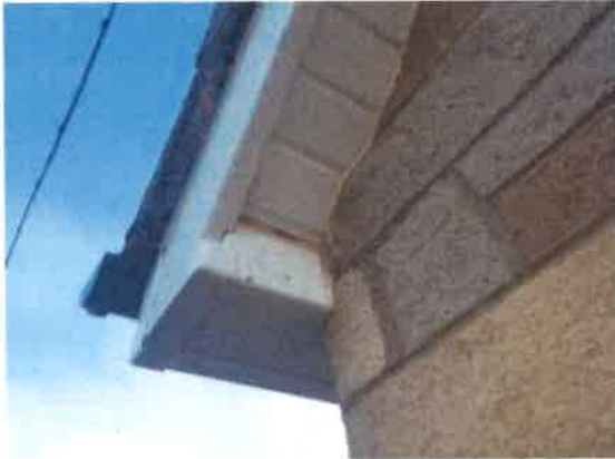
31 Possible asbestos cement at verge.
