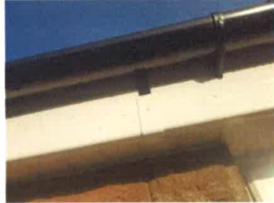
56 Overflow at fascia.
