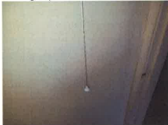
21 Water run off marks within Bathroom.
