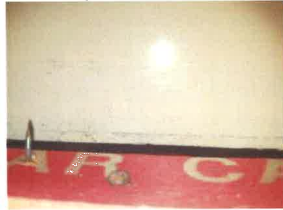
28 Gap at underside of skirting – unsealed.
