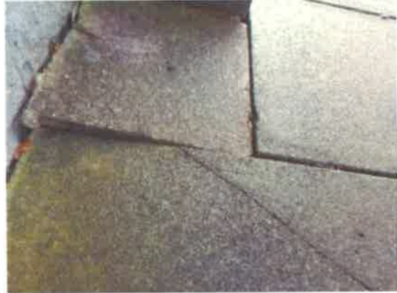
34 Defective concrete paving slabs.
