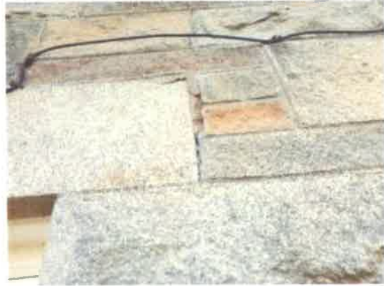
36 Cracking to pointing.
