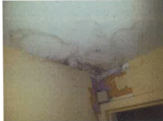
20 Water damage within bathroom.
