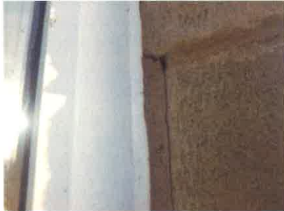
45 Cracking to pointing.
