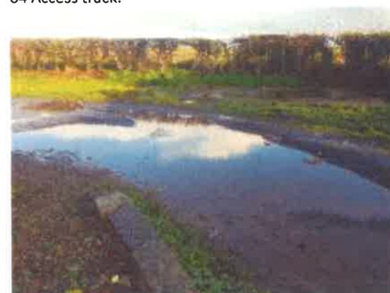
66 Potholing and water ponding
