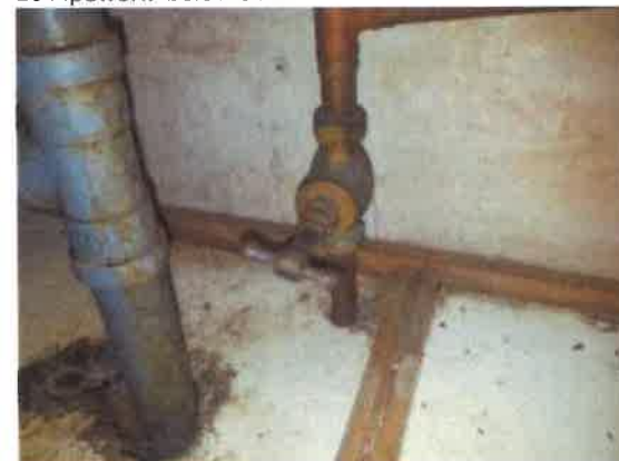
12 Water shut-off valve.
