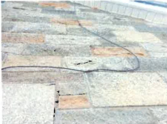
37 Cable clipped at gable.
