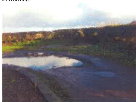
65 Potholing and water ponding.
