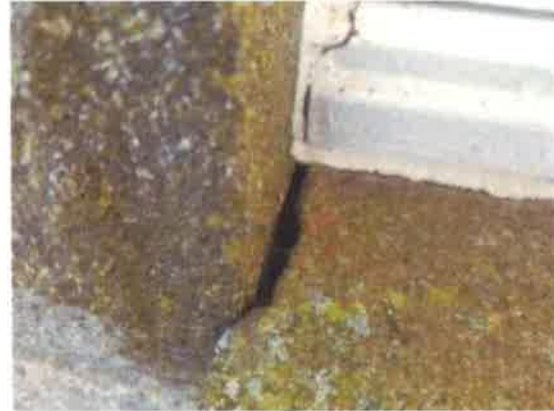
46 Open gaps at sills.
