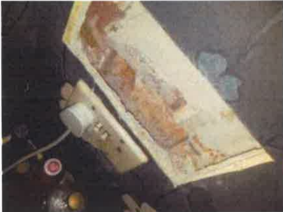
7 Damage adjacent to fireplace.
