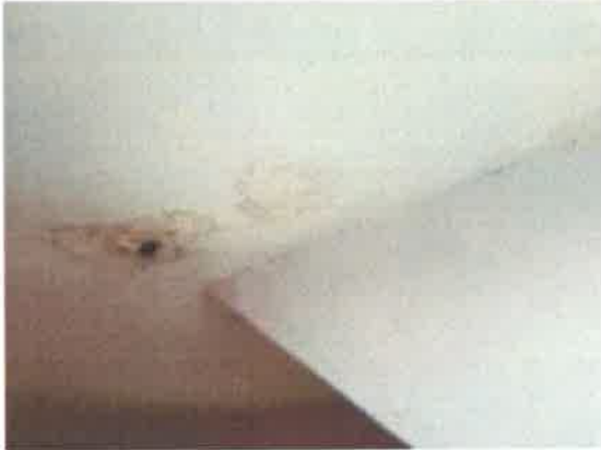
25 Water damage within Bedroom.
