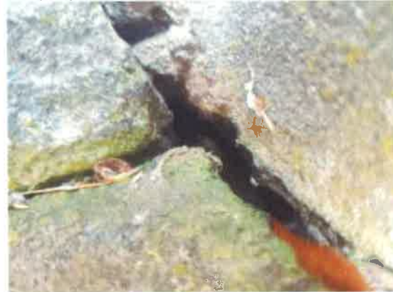
40 Close view of gap at gable steps.
