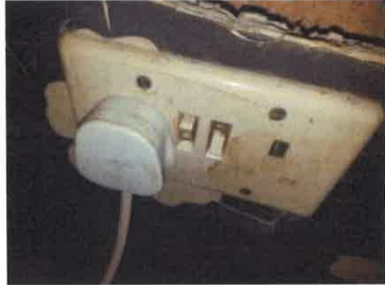
8 Socket outlet adjoining fireplace.
