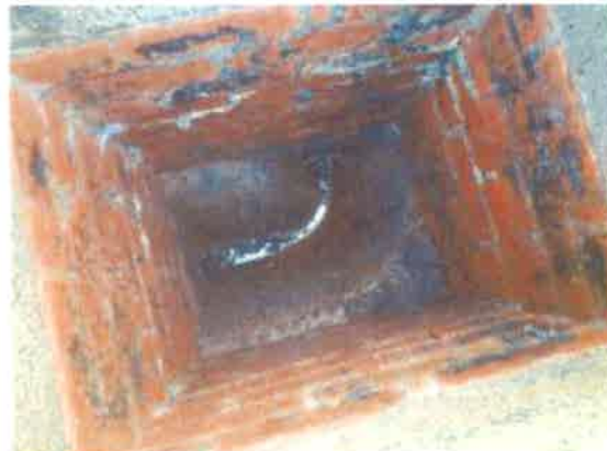
59 Impairment of drainage flow.
