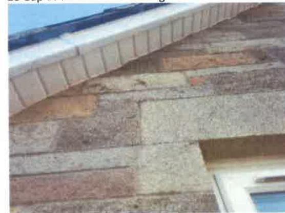
30 Possible asbestos cement at verge.
