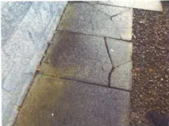
33 Defective concrete paving slabs.
