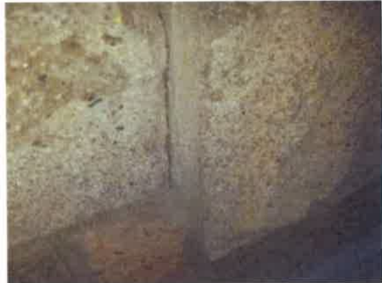
32 Cracking to pointing.
