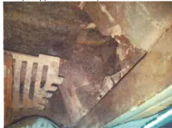
4 Damage within fireplace.
