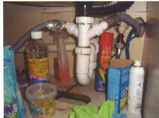
PLUMBING BENEATH KITCHEN SINK
