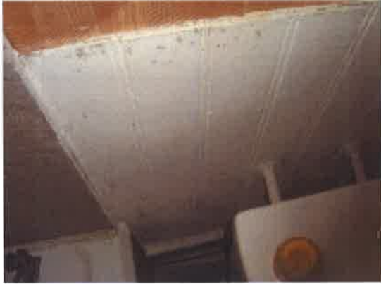
MOULD AT REAR OF WC
