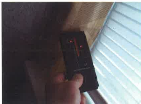
BATHROOM WINDOW – “DAMP”
