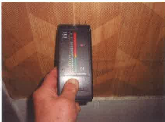
REAR WALL OF BATHRM – “DRY”
