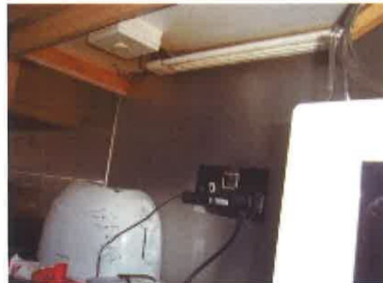
DOWNLIGHTS AT KITCHEN CPDS
