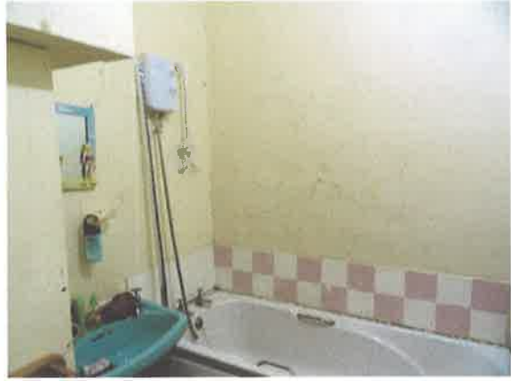
6. Missing shower screen
